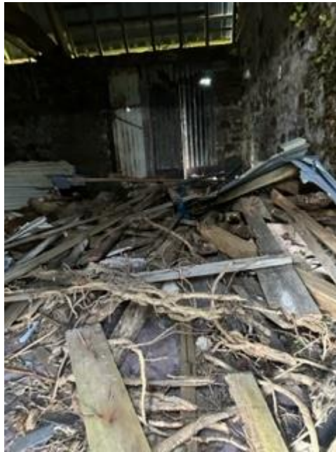
Figure 25 Debris to right hand room.
