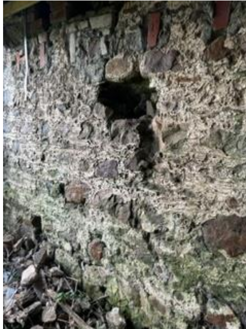
Figure 17 Internal deterioration to internal wall
