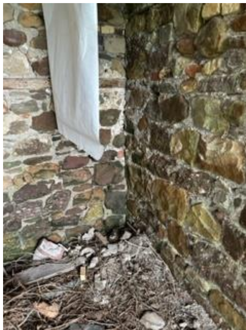
Figure 14 Cracking at junction of gable end and LH gable end elevation
