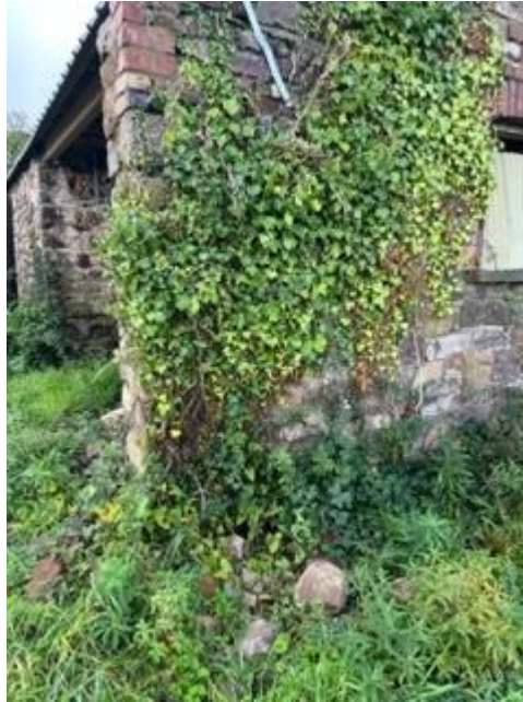
Figure 9 Close up of low-level masonry deterioration
