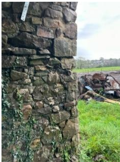
Figure 12 Deterioration to gable end - internally
