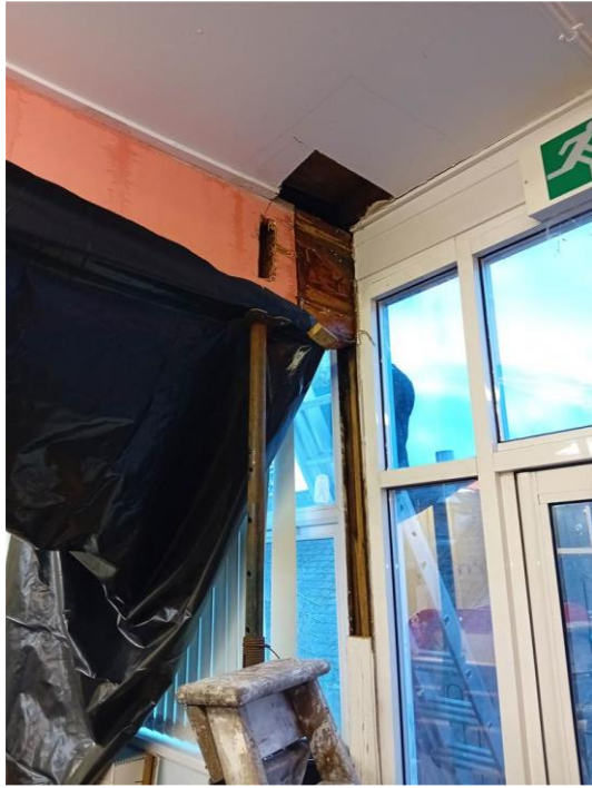
Above: 'dropped' beam with tarpaulin to contain water-ingress
