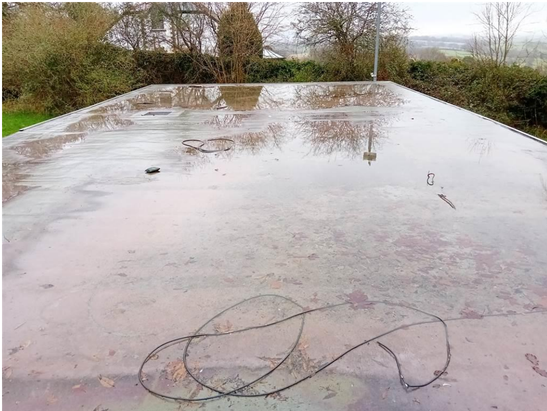
Left: Significant ponding on annexe roof (2024)
