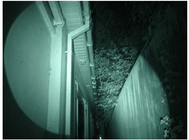
Photo 6. The southwestern elevation of the main building of the day centre at the darkest point of the survey on the 4 th June 2025 from NVA location 3.
