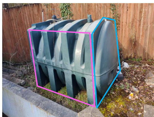
Photo 16. The northeastern (blue) and southeastern (pink) elevations of the fuel storage container.
