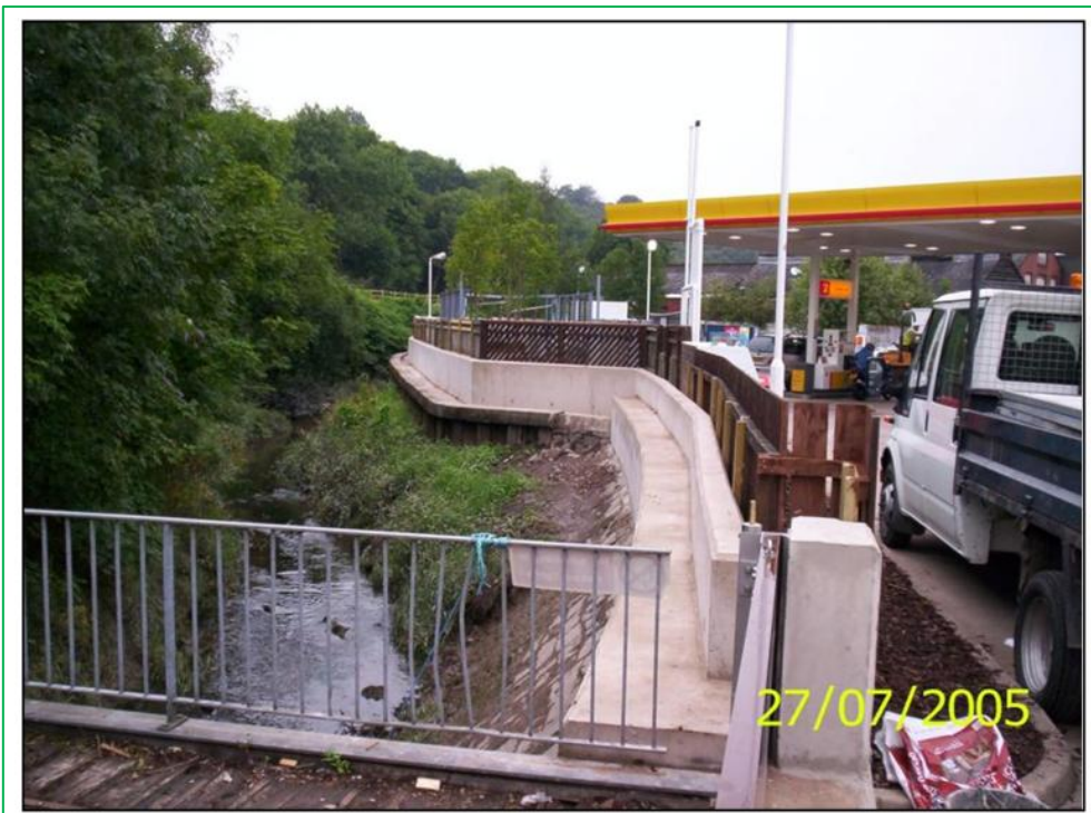
Figure 5 - Malpas Brook Flood Wall
