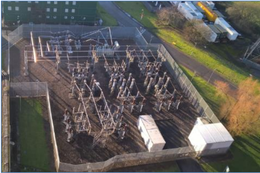
Figure 7 Existing Uskmouth 132kV substation
