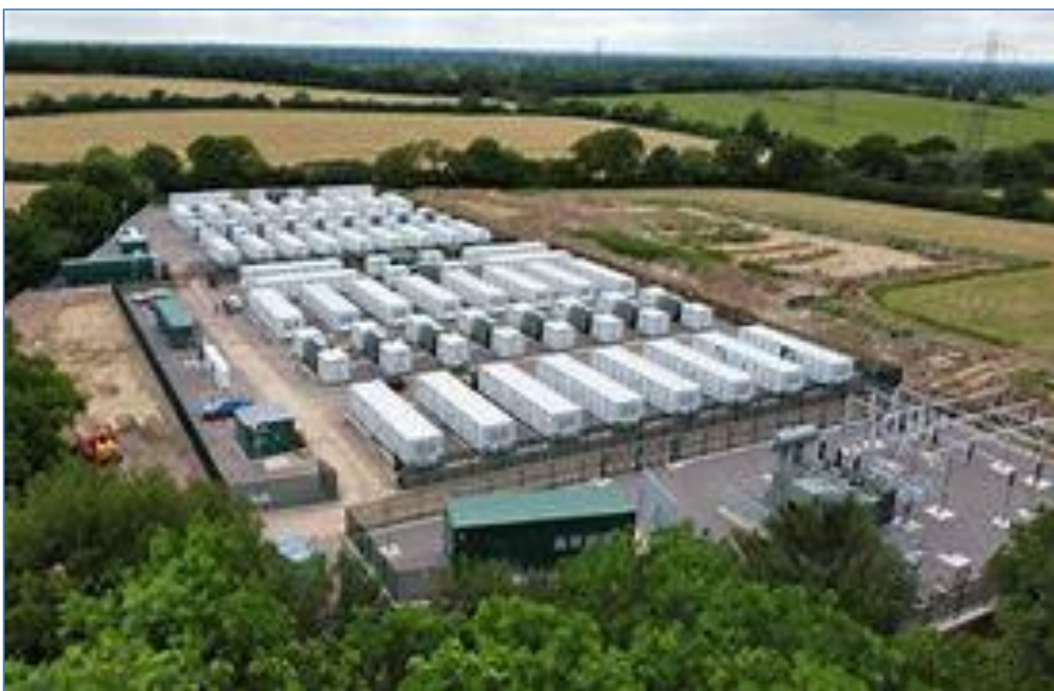
Figure 5 Example of BESS project
