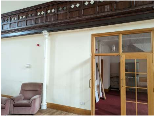
8. Cast iron columns supporting former gallery and entrance to offices and WCs
