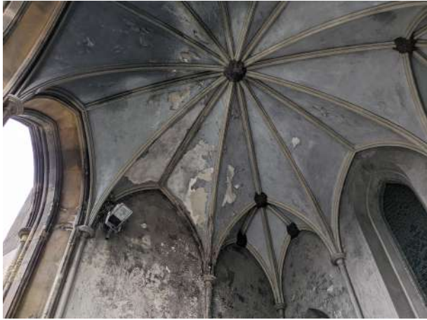
2. The smoked damaged entrance porch
