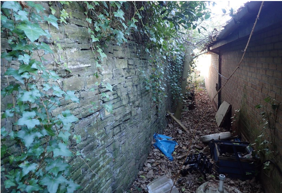
Image EDP 2: View of the original boundary wall to the rear of the healthcare centre.
