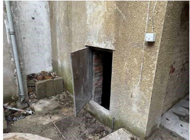
Entrance to cellar from designated commercial area, locked and for Landlord use only
