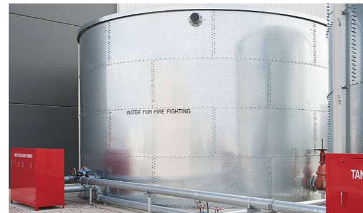
Typical sprinkler tank
