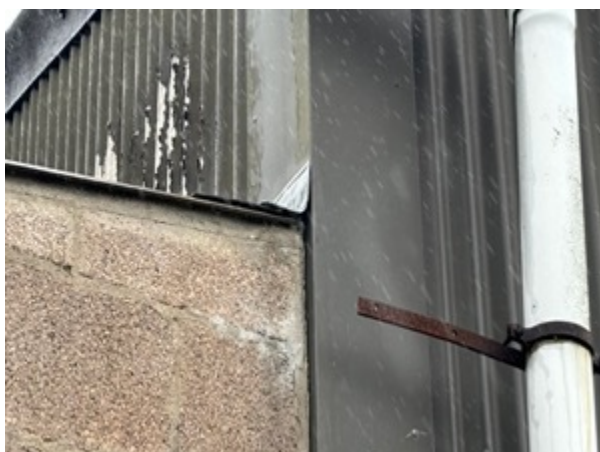
Photo 11: Raised Lead Flashing
