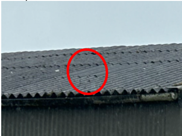
Photo 3: Roof of The Barn (Gaps in The Roof Circled)
