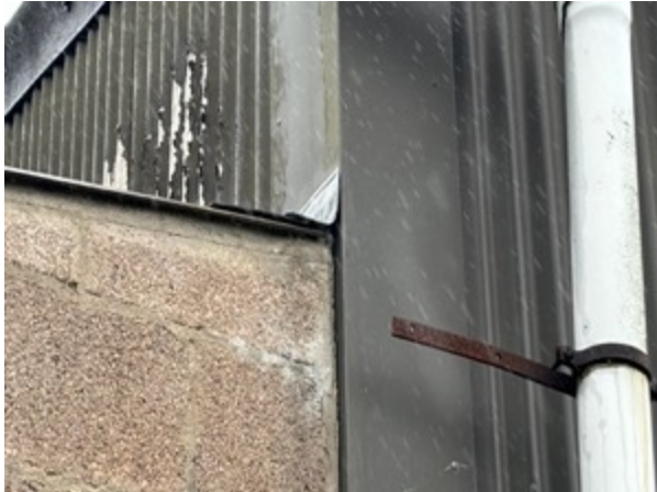
Photo 11: Raised Lead Flashing
