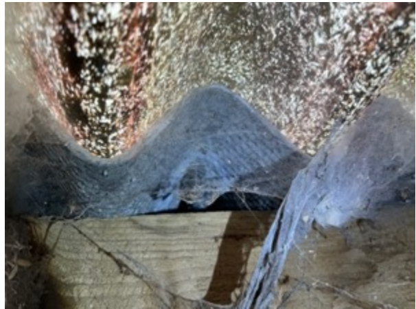
Photo 4: Gaps Underneath The Plastic Sheeting
