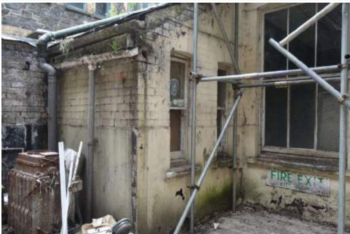
Plate 22: View looking SE towards the W elevation of the one storey extension.
