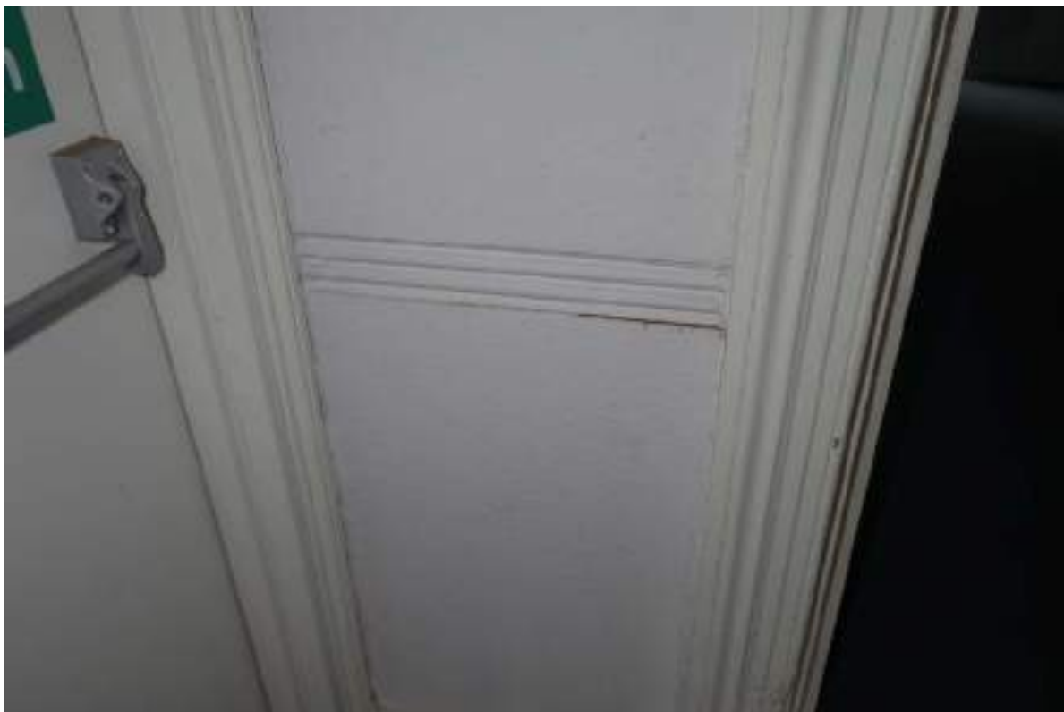
Plate 80: View looking NW in FF Room 2, towards a section of dado rail.
