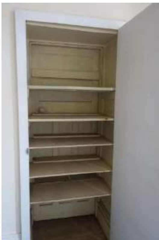
Plate 118: View looking ESE towards the cupboard between FF Room 12c and FF Room 9.
