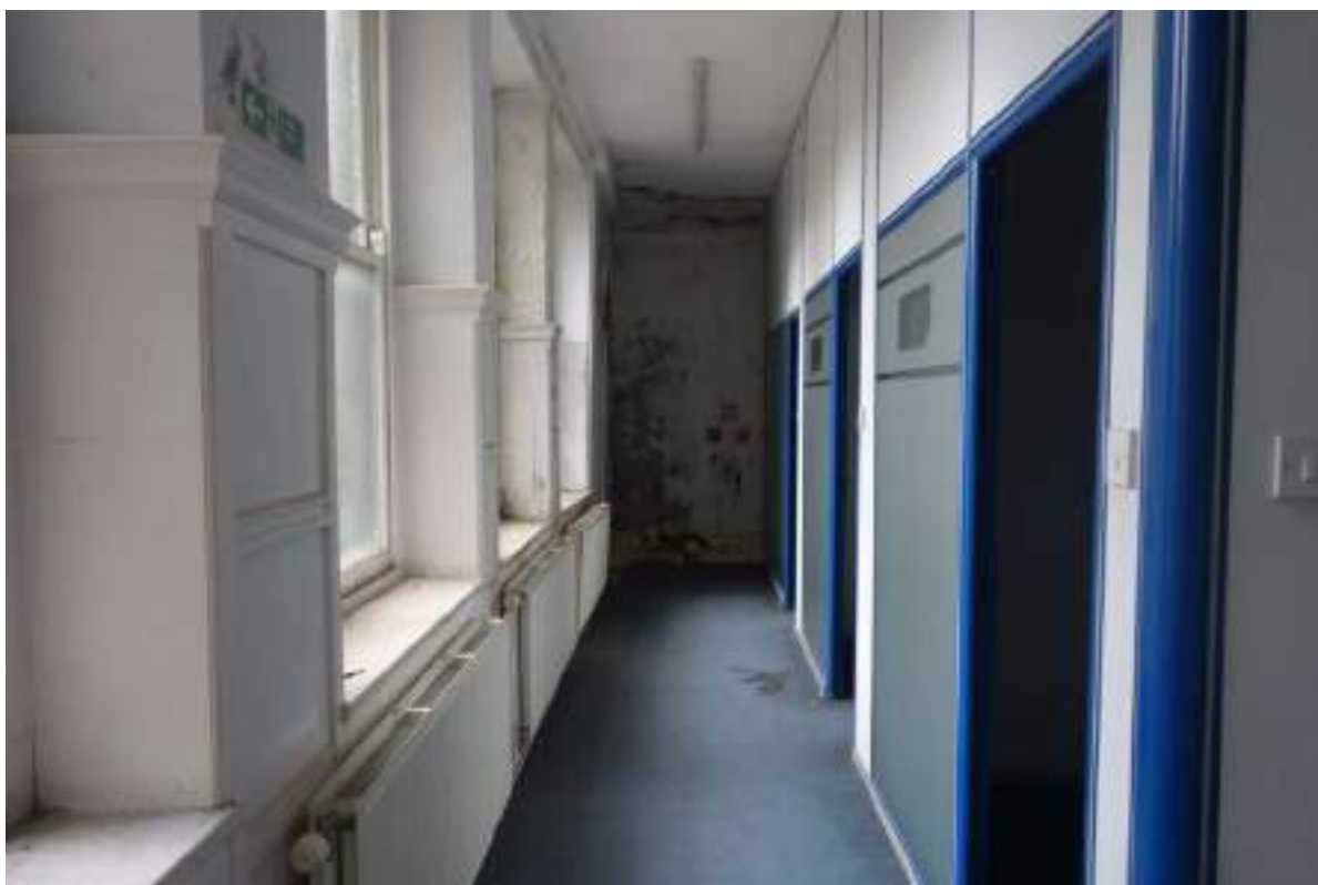
Plate 83: View looking NNW in FF Room 4, showing the sash windows and wooden panelling between.
