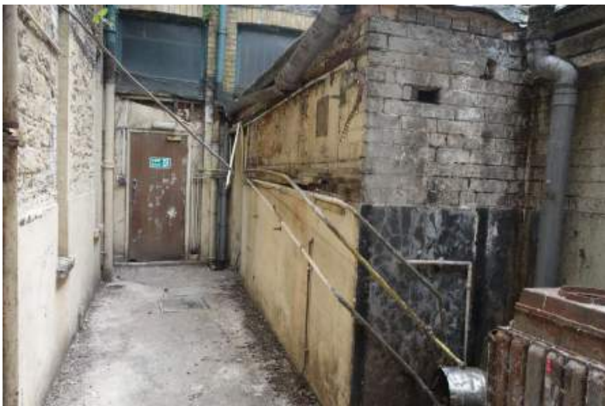
Plate 21: View looking E across the courtyard (GF Room 8), along the one storey extension.
