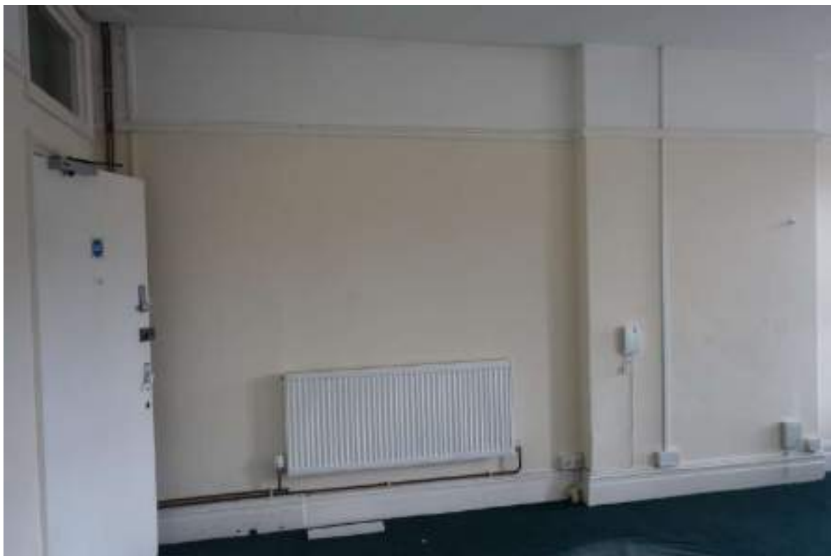
Plate 197: View looking ENE in TF Room 10, showing the picture rail and the window above the door.
