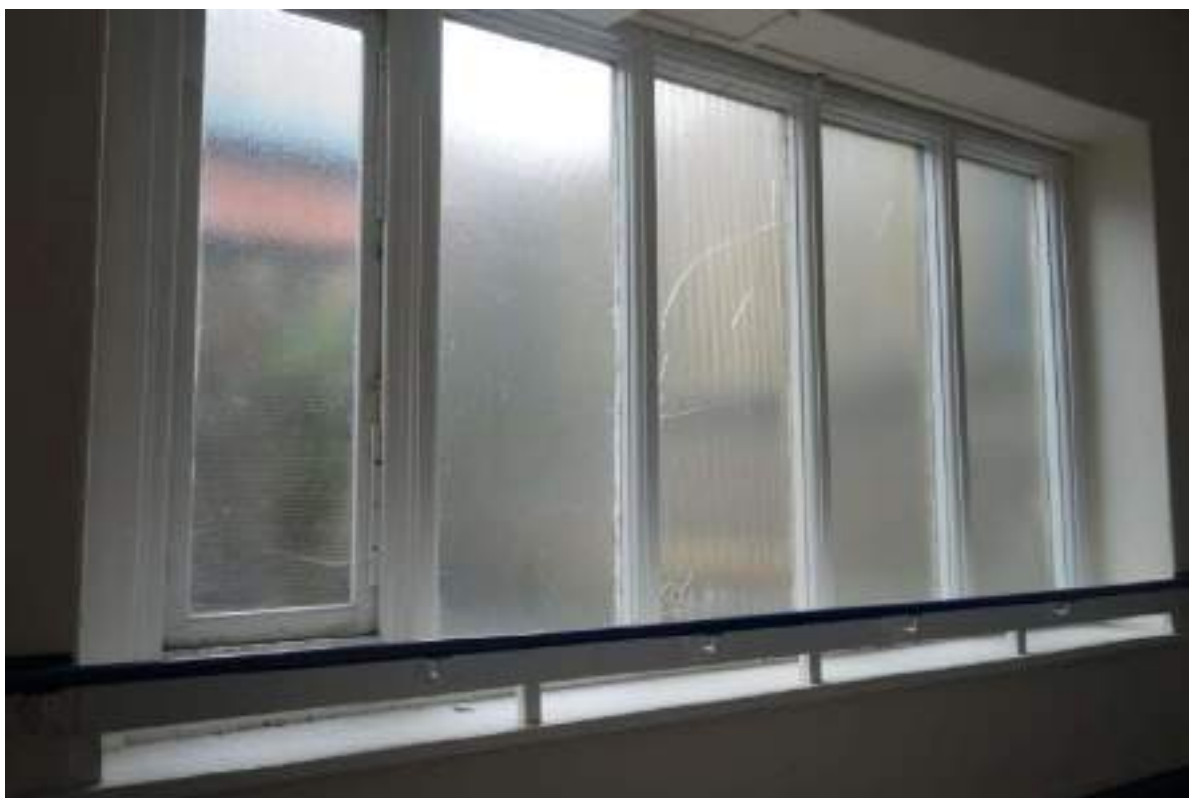
Plate 75: View looking NE across the windows of the main staircase (GF to FF).
