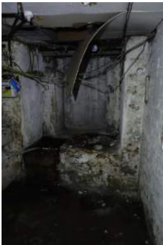
Plate 62: View looking N in the basement's fourth compartment, in the NW sub-compartment.
