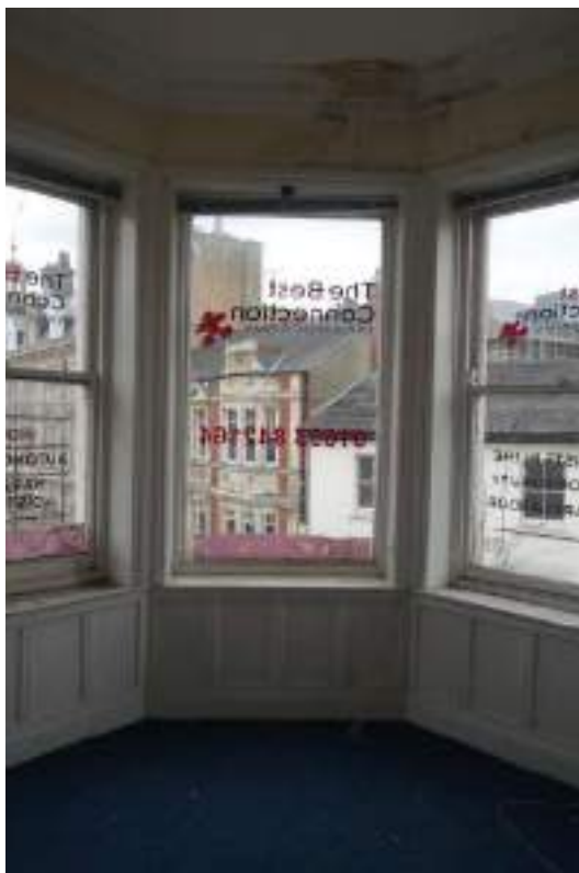
Plate 145: View looking NE in SF Room 3c, towards the windows of the corner bay and the wooden panelling beneath.
