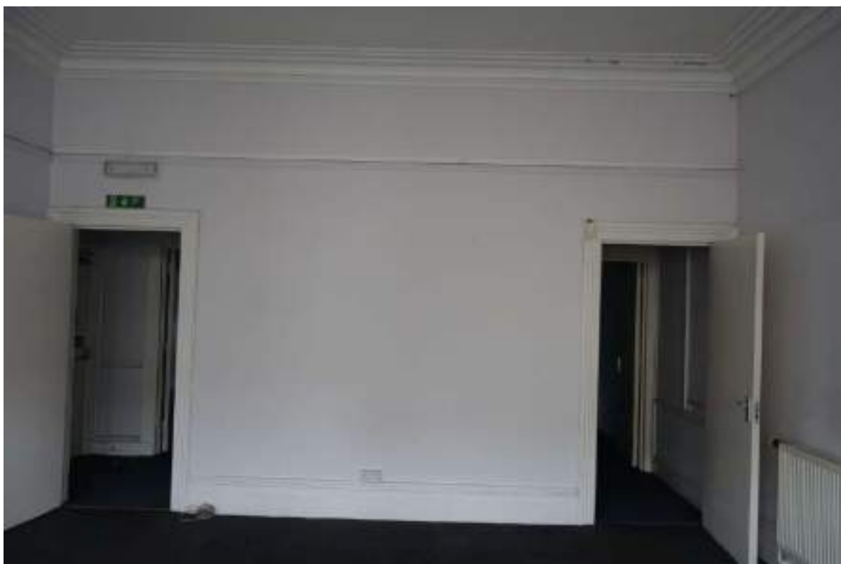
Plate 106: View looking N in FF Room 9, towards the two doorways with architraves, showing the picture rail.
