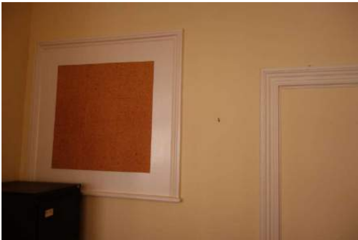
Plate 127: View looking S in FF Room 15a, towards a blocked interior window and doorway.
