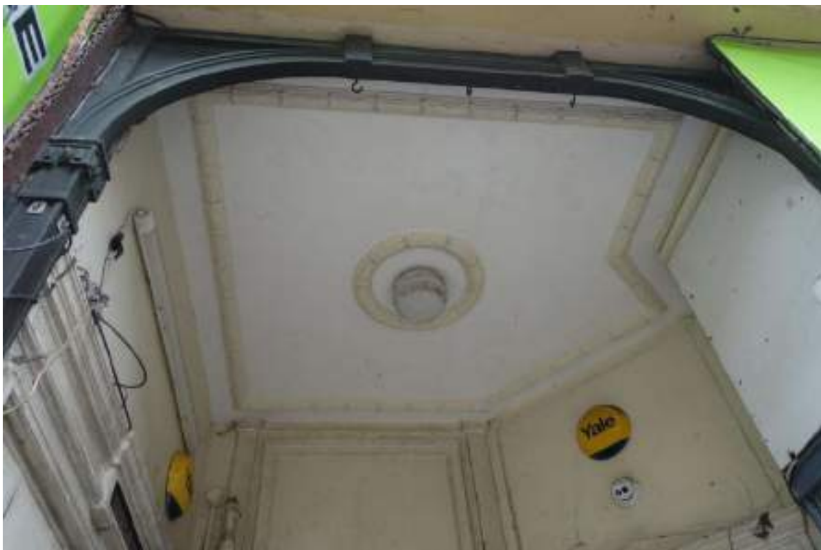
Plate 64: View looking N and up in GF Room 21, towards the porch's ceiling mouldings.
