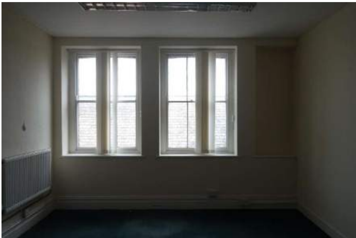
Plate 184: View looking N in TF Room 4, towards two sash windows and half of a boarded-up window recess.
