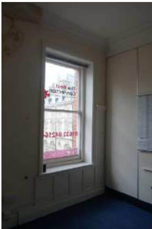
Plate 147: View looking ENE in SF Room 3e, towards a sash window with wooden panelling beneath.
