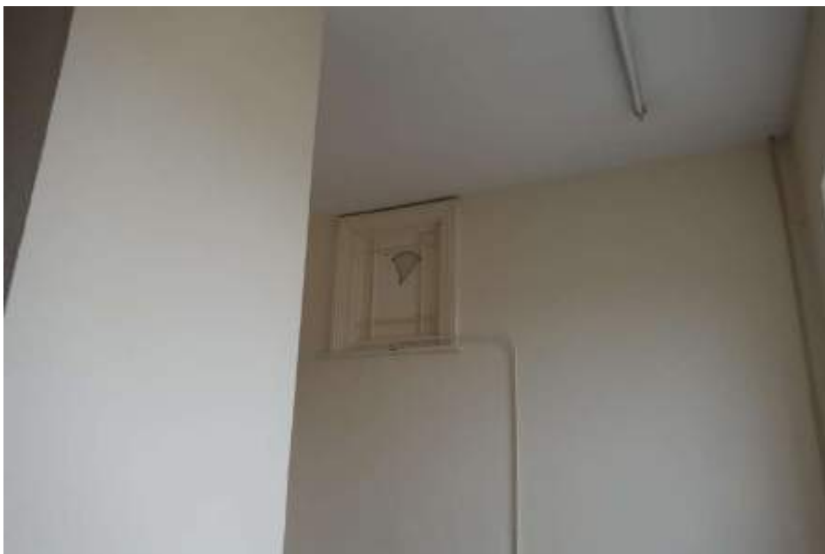
Plate 177: View W and up from the main staircase's middle flight, towards a blocked interior window.
