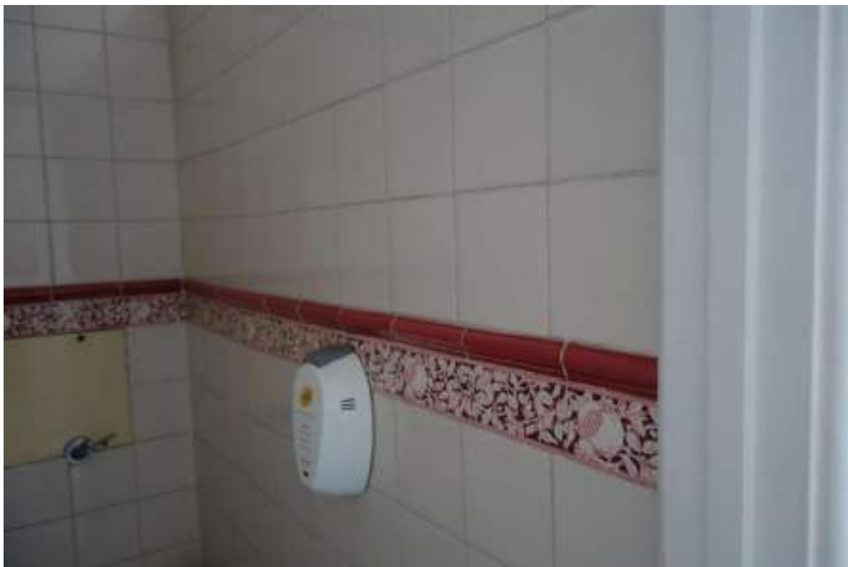
Plate 99: View looking NE in FF Room 7, showing an area of wall tiling.
