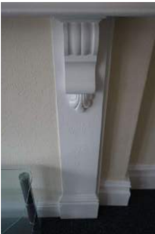
Plate 156: View looking W, towards the corbel of the mantel piece in SF Room 6.
