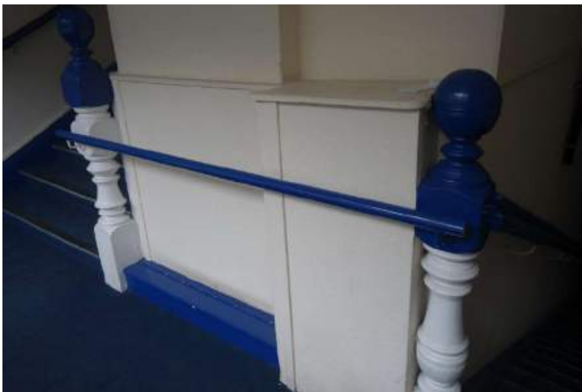
Plate 73: View looking SSE, towards two newel posts on the middle landing of the main staircase (GF to FF).
