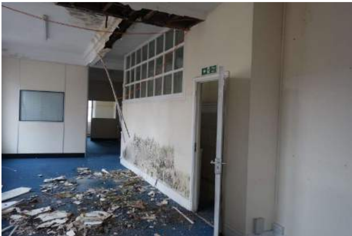
Plate 150: View looking SSW in SF Room 4, towards the partition wall with upper windows of the FF to SF E-bay staircase and the SF to FF E-bay staircase (SF Room 5).
