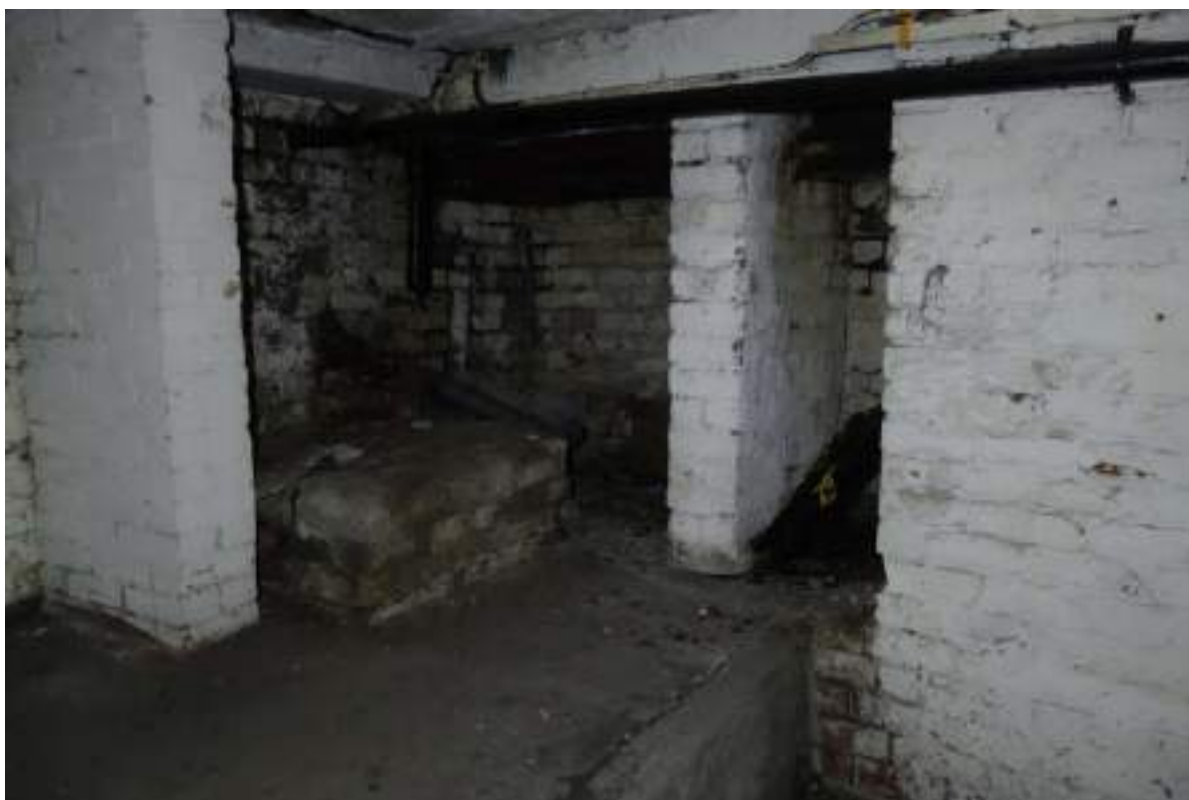
Plate 63: View looking NE in the basement's fourth compartment, in the NE sub-compartment.
