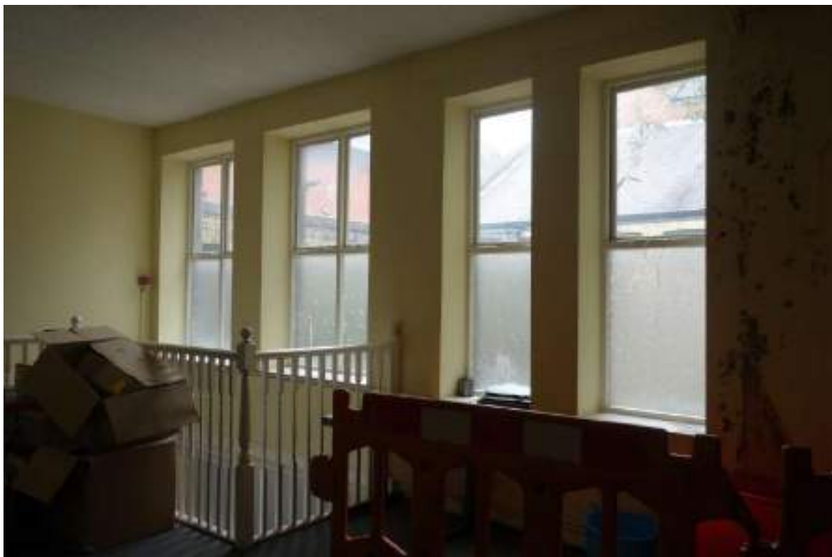
Plate 125: View looking NE in FF Room 15, towards the windows and GF to FF W-bay staircase.
