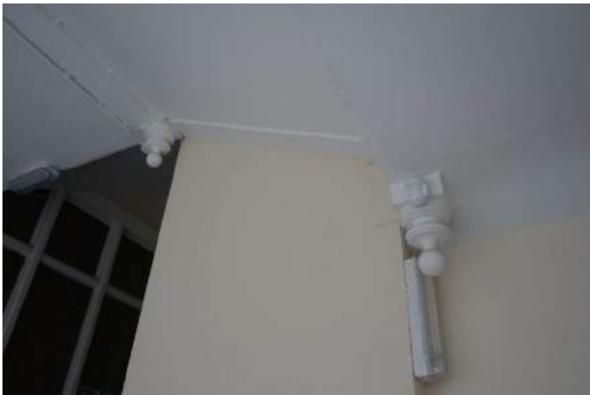
Plate 74: View looking SE and up, towards two pendants on the middle landing of the main staircase (GF to FF).
