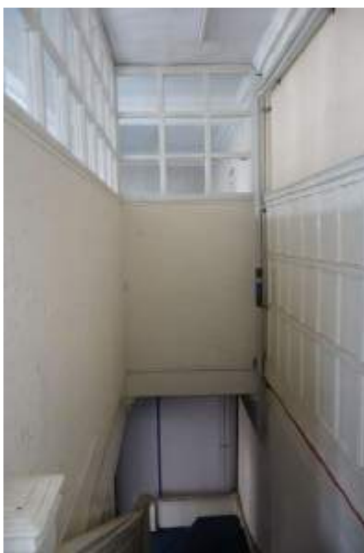
Plate 104: View looking S, showing the wooden panelling and interior windows associated with the FF to SF E-bay staircase.
