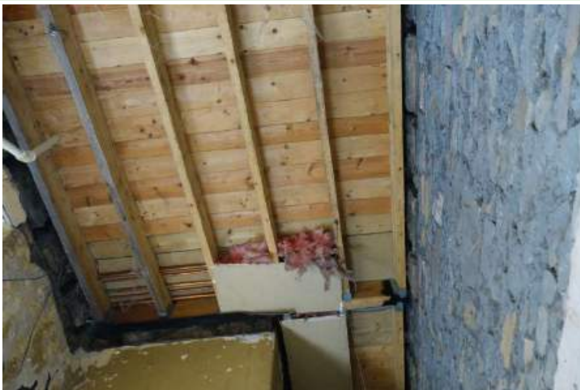
Plate 33: View looking WNW and up in GF Room 10, showing the stone of the wall.
