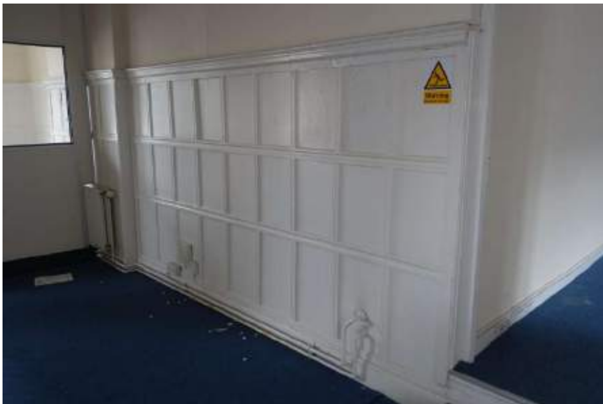
Plate 141: View looking NW in SF Room 3a, towards a large section of wooden panelling.
