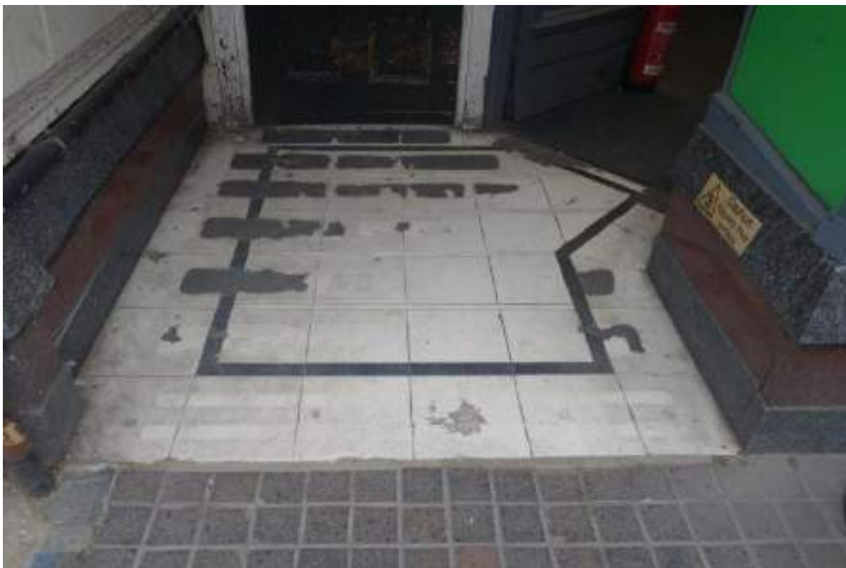
Plate 65: View looking N and down in GF Room 21, towards the porch's floor tiles.
