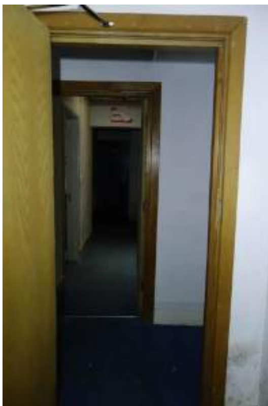
Plate 47: View looking N in GF Room 16b, across GF Room 17 and towards GF Room 18.
