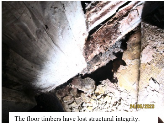
The floor timbers have lost structural integrity.
