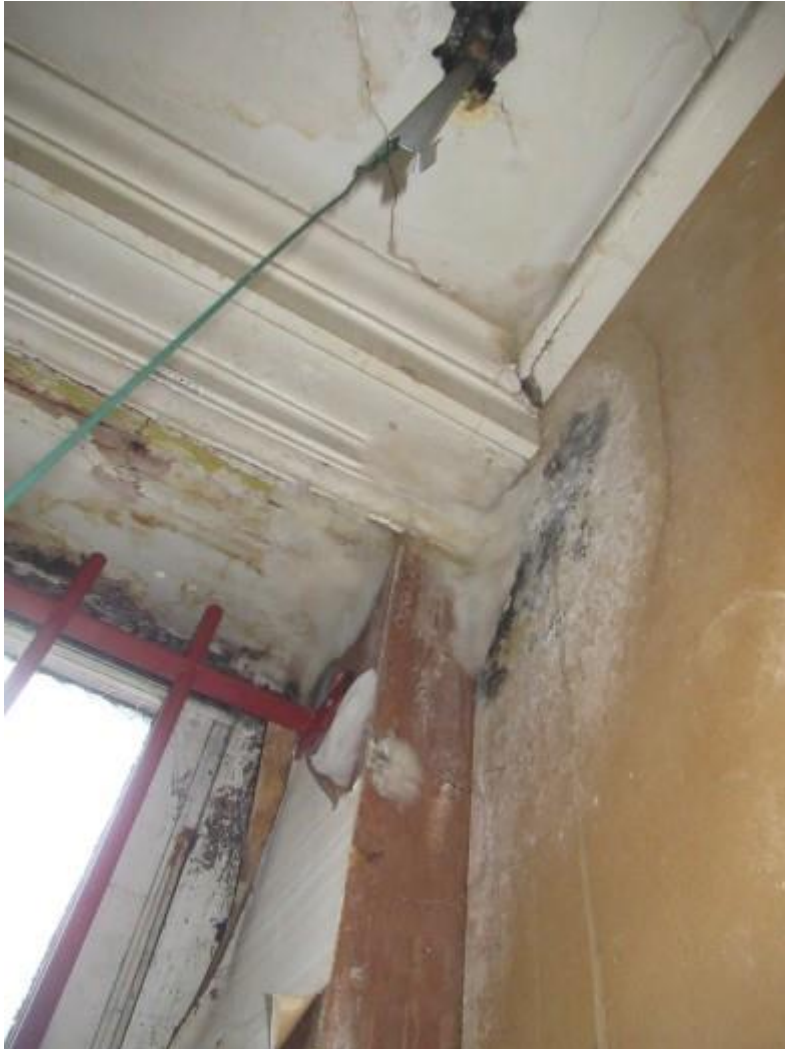
Dry rot and fungal growth above the suspended ceiling to the left hand side store room to the ground floor right hand side unit.
