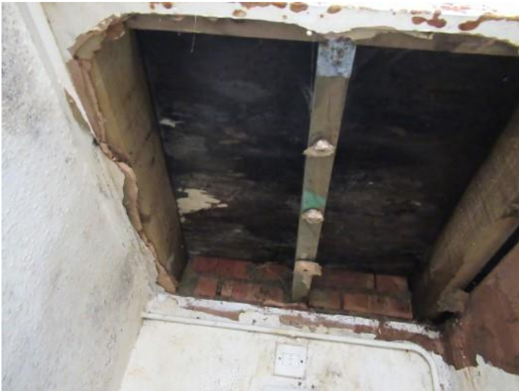
Underside of the flat roof above the WC accommodation. There are areas of rot and decay affecting timbers consistent with water ingress.
