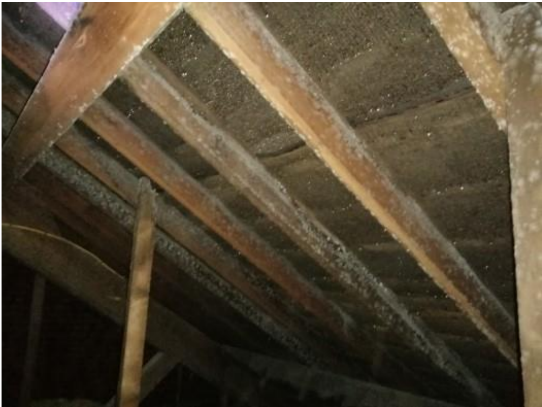
Further illustration of moisture to underside of sarking felt and condensation to timbers.
