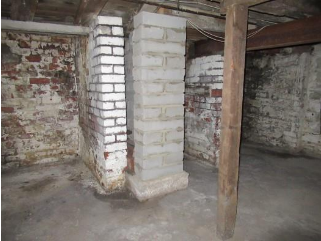
Basement area where below the ground floor right hand unit. The photograph shows evidence of past repair and strengthening to the underside of the floor to include steel and concrete beams providing intermediate support of the floor timbers. The photograph also shows a concrete block pillar providing intermediate support.
