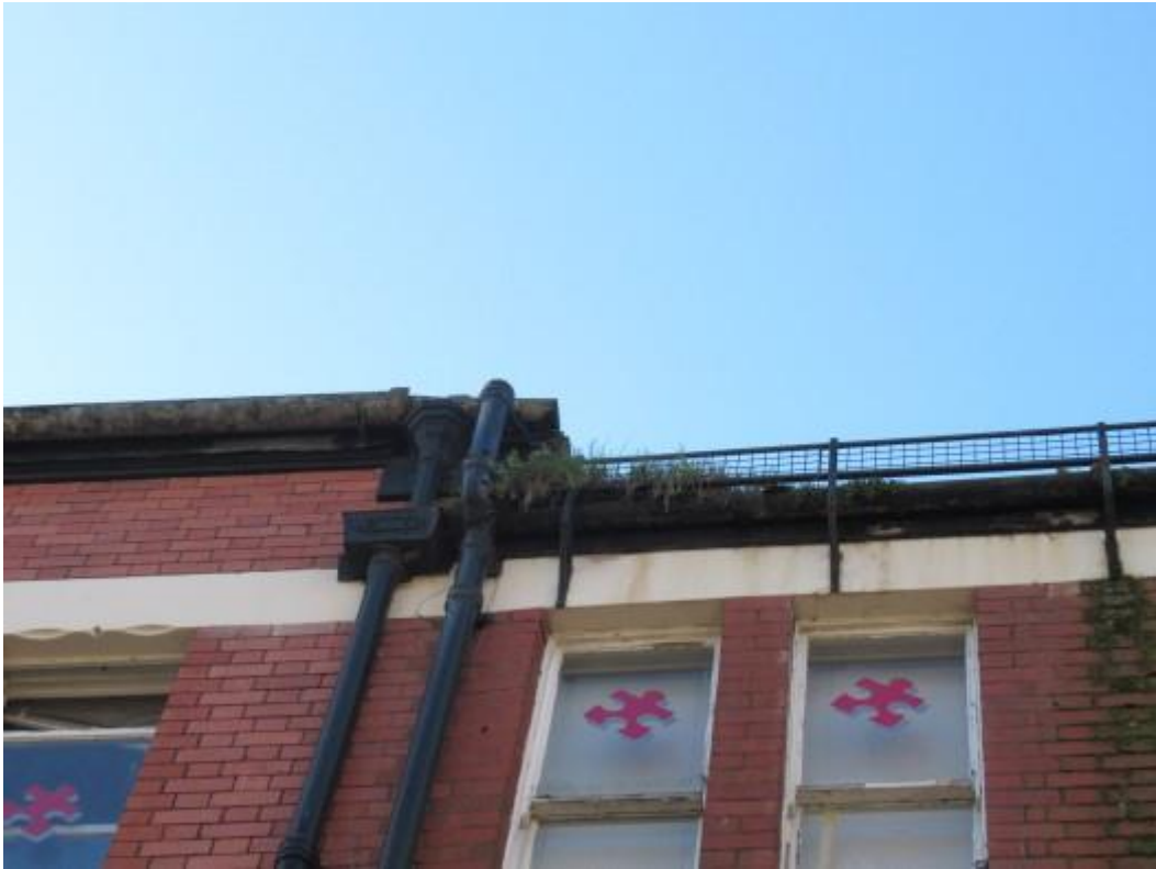
Further illustration of typical blockage and vegetation within the guttering.
