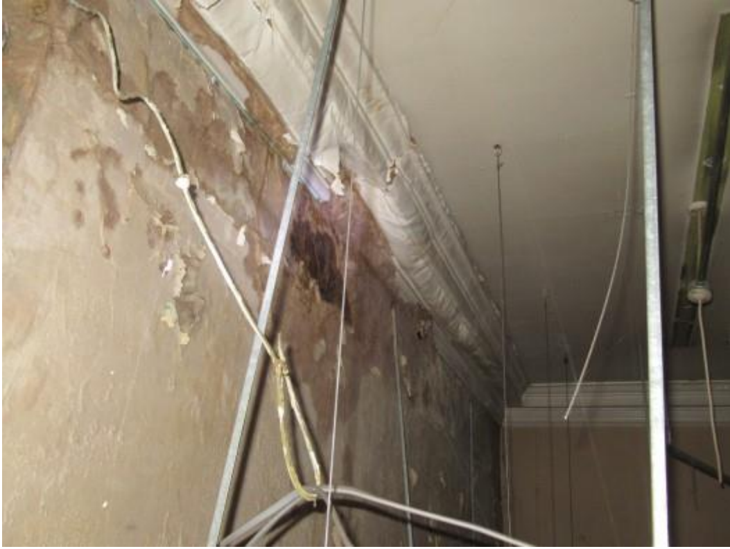
View above the ceiling to the kitchen area to the right hand side unit. There is extensive dry rot to this area. Substantial replacement of timbers and specialist treatment work will be required.
