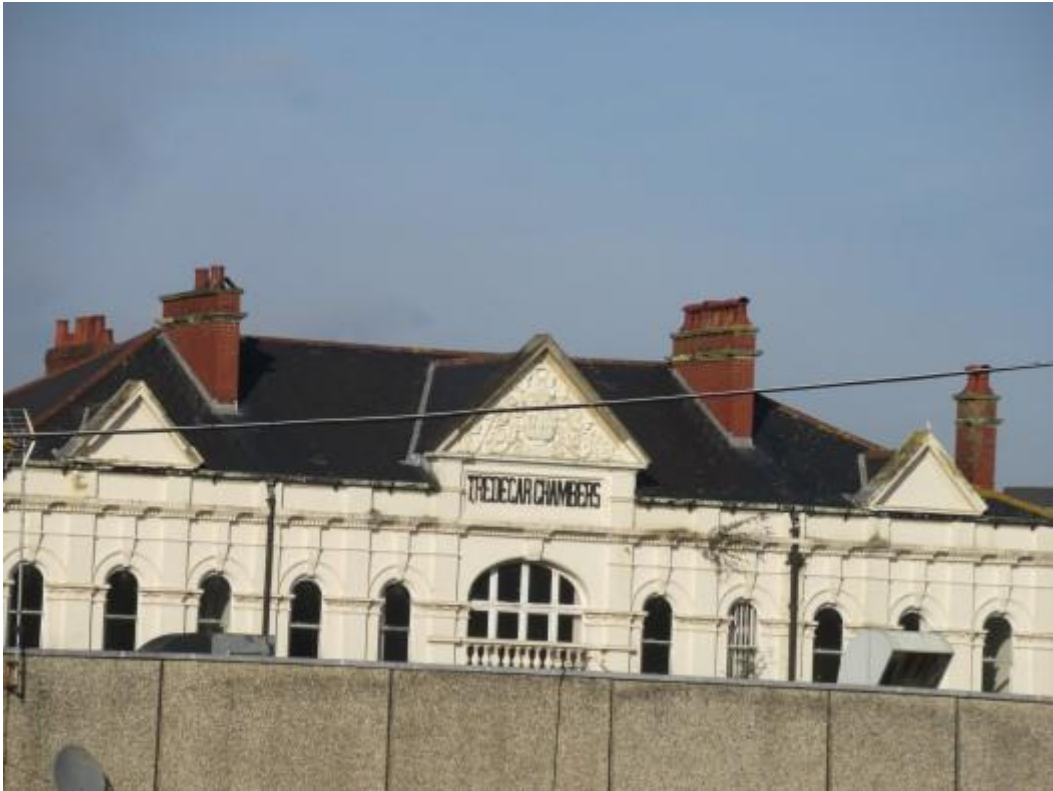
Roof slopes where extending to the front of the property. The photograph shows three feature gable roofs with lead valley details formed between the gable roofs and front main roof slopes.
