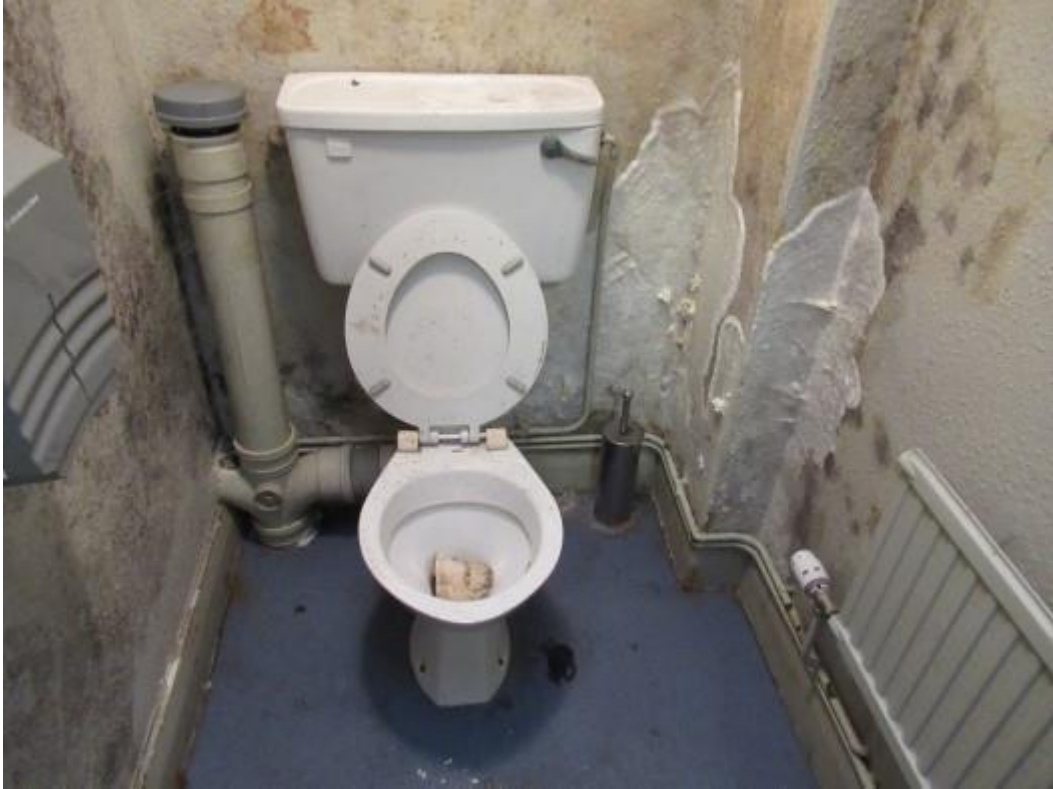
Further illustration of rot within ground floor WC accommodation.
