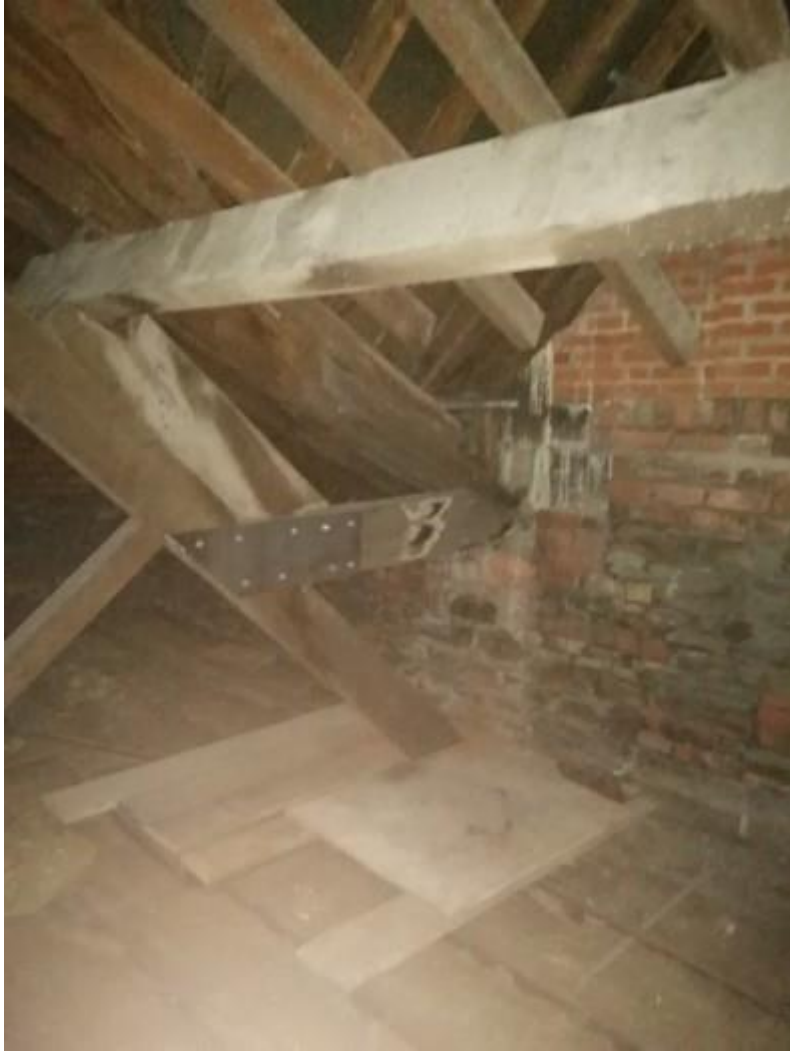
Further illustration of past repair towards the central roof area where extending towards the front gable.
