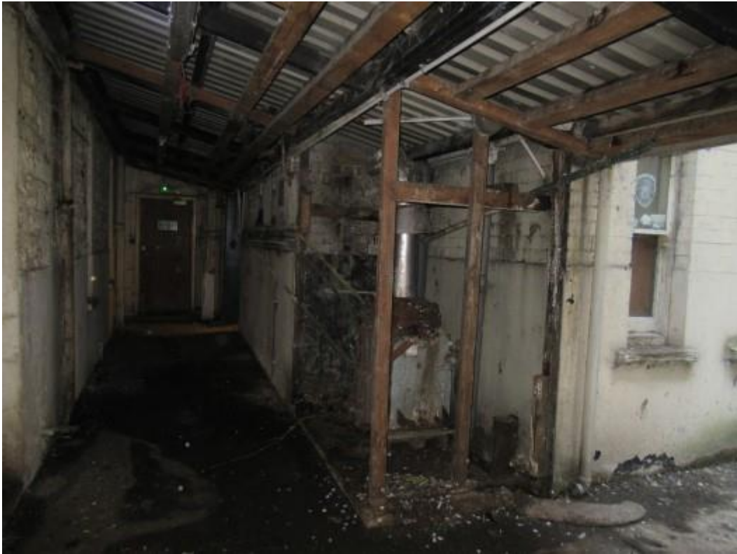
Further illustration of the covered area to the rear with water ingress noted.
