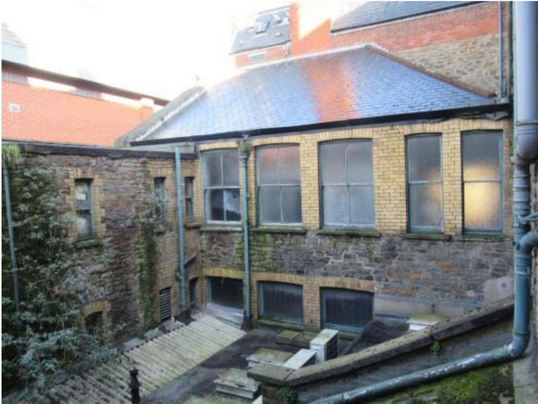
Further illustration of walling to the rear. Past re-pointing work has been carried out. The photograph shows the areas of brickwork detailing. No significant damage was noted.
