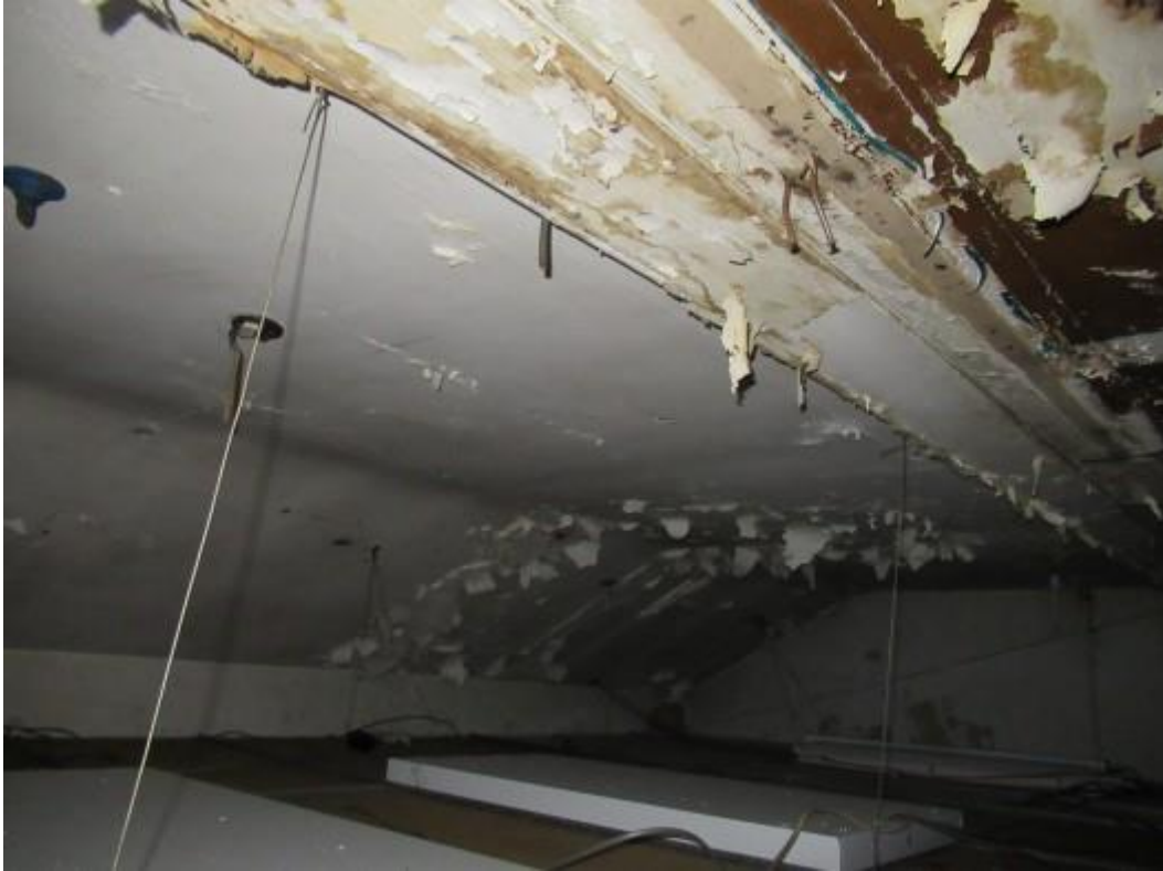
View above the suspended ceiling. An older lath and plaster ceiling is noted. This has deteriorated with age.
