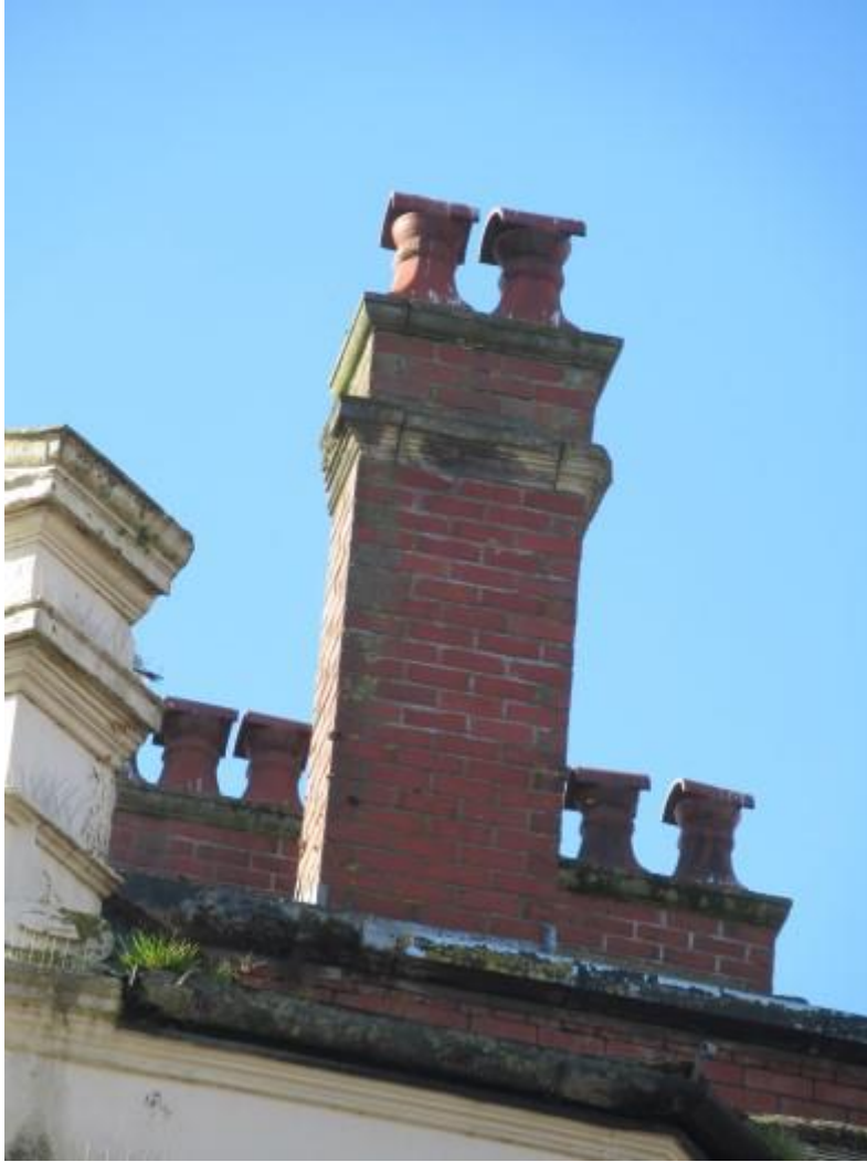
Further illustration of typical chimney stack to the right hand side of the property as viewed from ground level.
