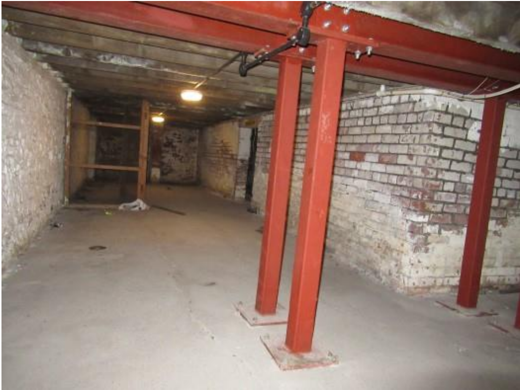
Further illustration of basement area with more recently installed steel framework noted. This provides support to the underside of the stair area.
