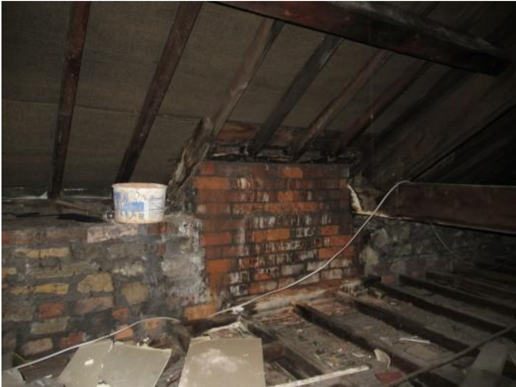
Further illustration of timbers to the right hand side of the roof with more extensive rotten timbers around the side chimney stack noted.
