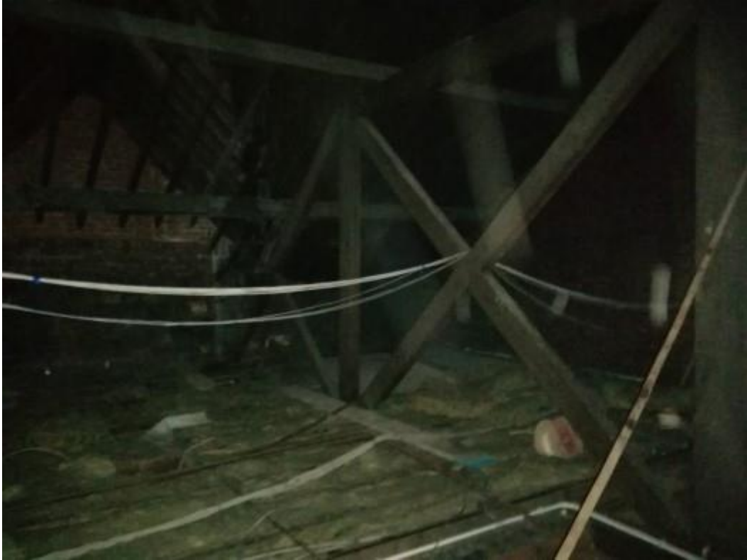
Central roof void. The photograph shows principal trusses providing support of the rafters. The photograph shows the roof as viewed towards the front of the property with the front central gable wall noted.
