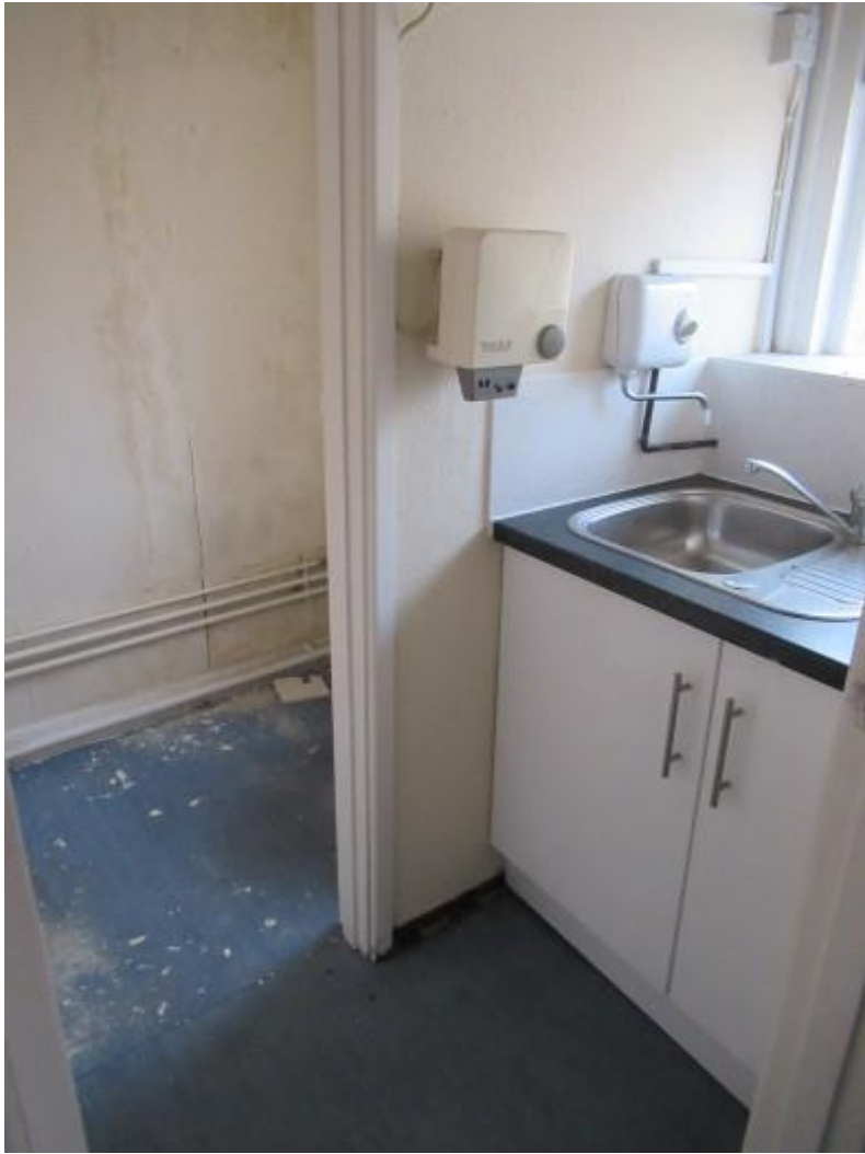
Typical condition of sink unit to first floor accommodation.
