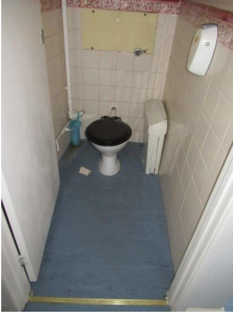
Typical condition of sanitary accommodation to the first floor.
