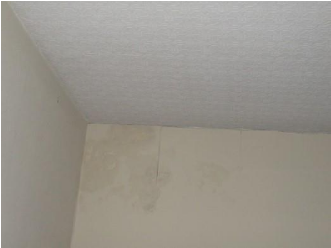
Damp affected and damaged plaster finishes to the kitchen accommodation to the rear of the first floor left hand side unit. This is below the flat roof area above.
