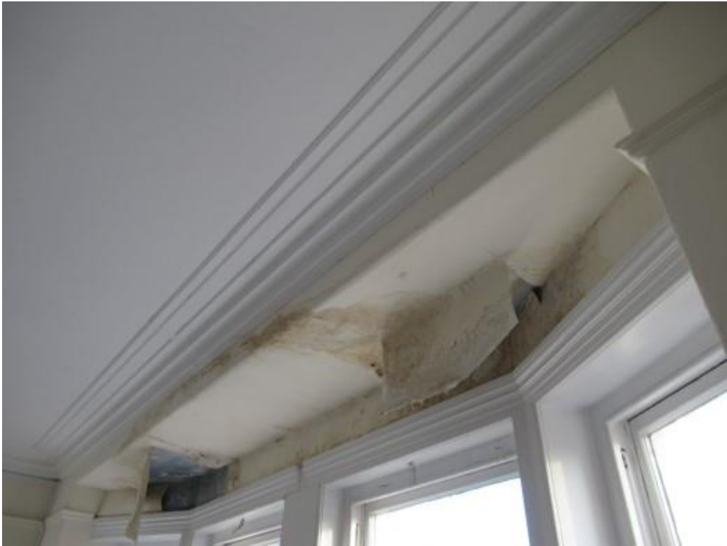
Damaged ceiling and water ingress to bay window area to the first floor to the front of the property. There is similar damp staining and damage to finishes to the bay windows throughout the property.
