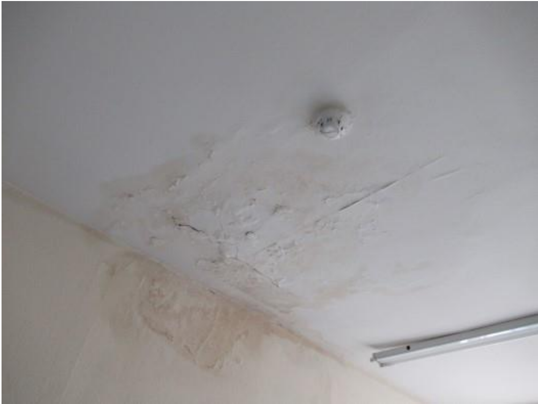
Typical damp staining to upper floor accommodation consistent with water ingress at the base of the chimney stack. This has caused damage to the wall and ceiling finishes.
