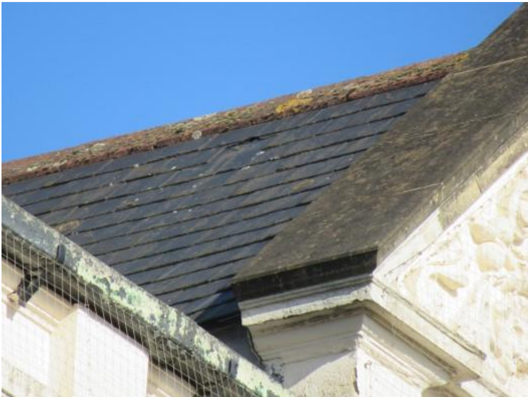
Failed slate to the front elevation of the property where extending to the front principal gable.
