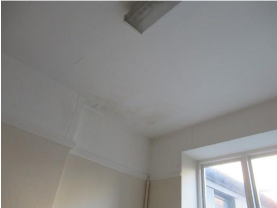
Damp affected and damaged wall and ceiling finishes to the first floor. This is consistent with leaking and overflowing rainwater goods externally.
