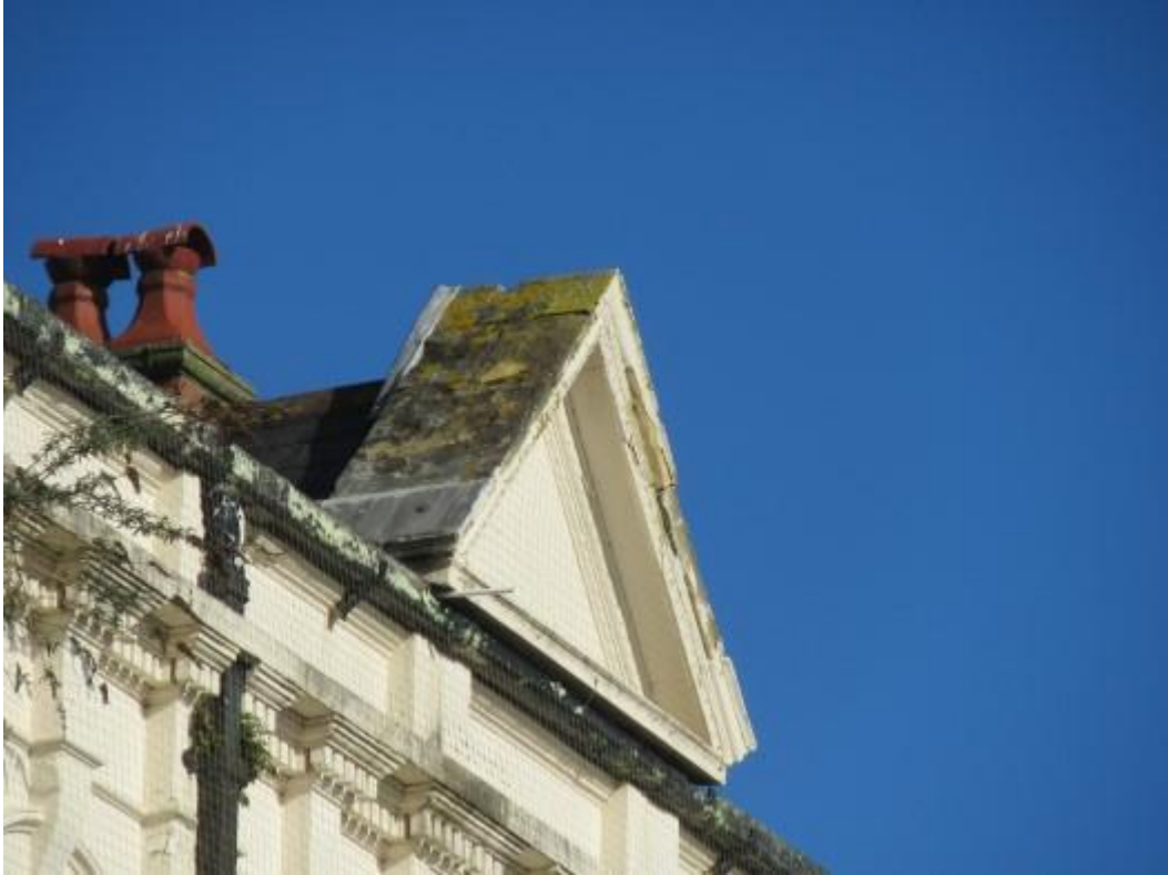
Right hand side gable with spalling, damage and general deterioration evident. Repair and upgrading works are required.
