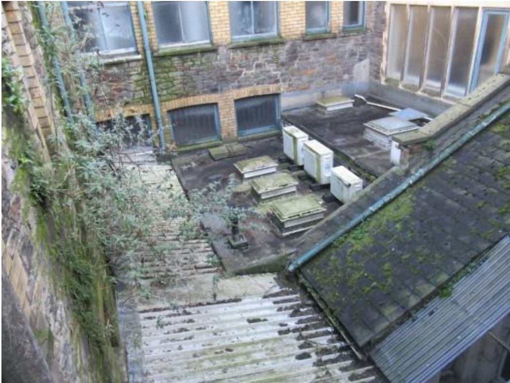
Further illustration of roofs to the rear with the lower level flat roof area noted.
