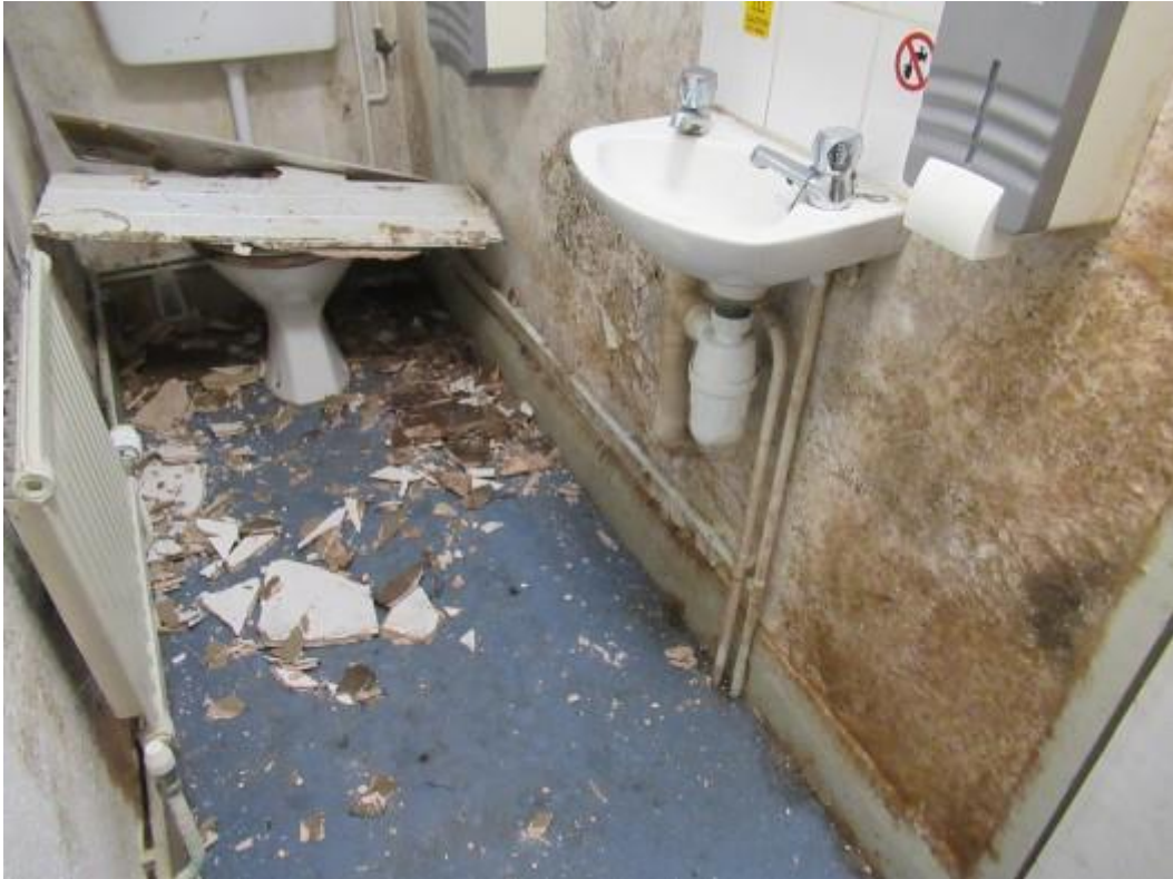
Rot within timbers to the WC accommodation to the rear.
