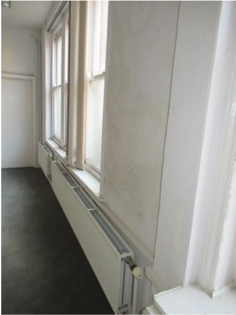
Typical damp affected and damaged plaster finishes consistent with water ingress.
