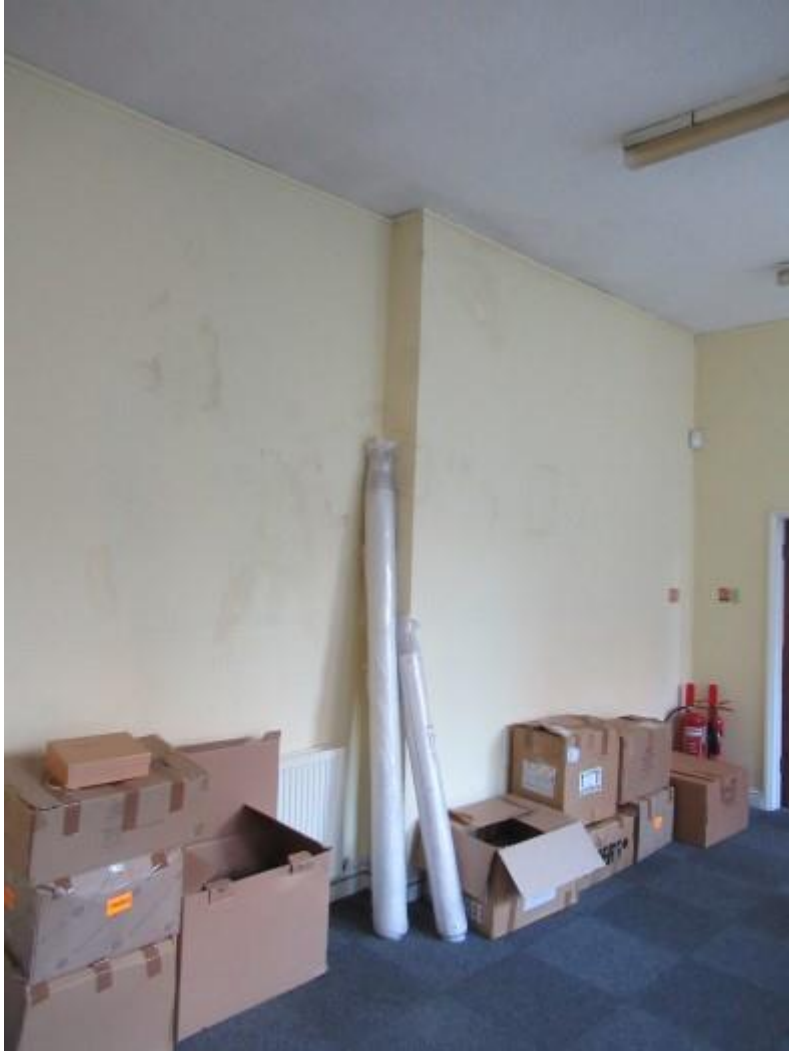
First floor accommodation to the left hand side of the property. The photograph shows damp staining of the side wall. This is below the parapet gutter detail formed between the left hand side lower level roof area and lead guttering.
