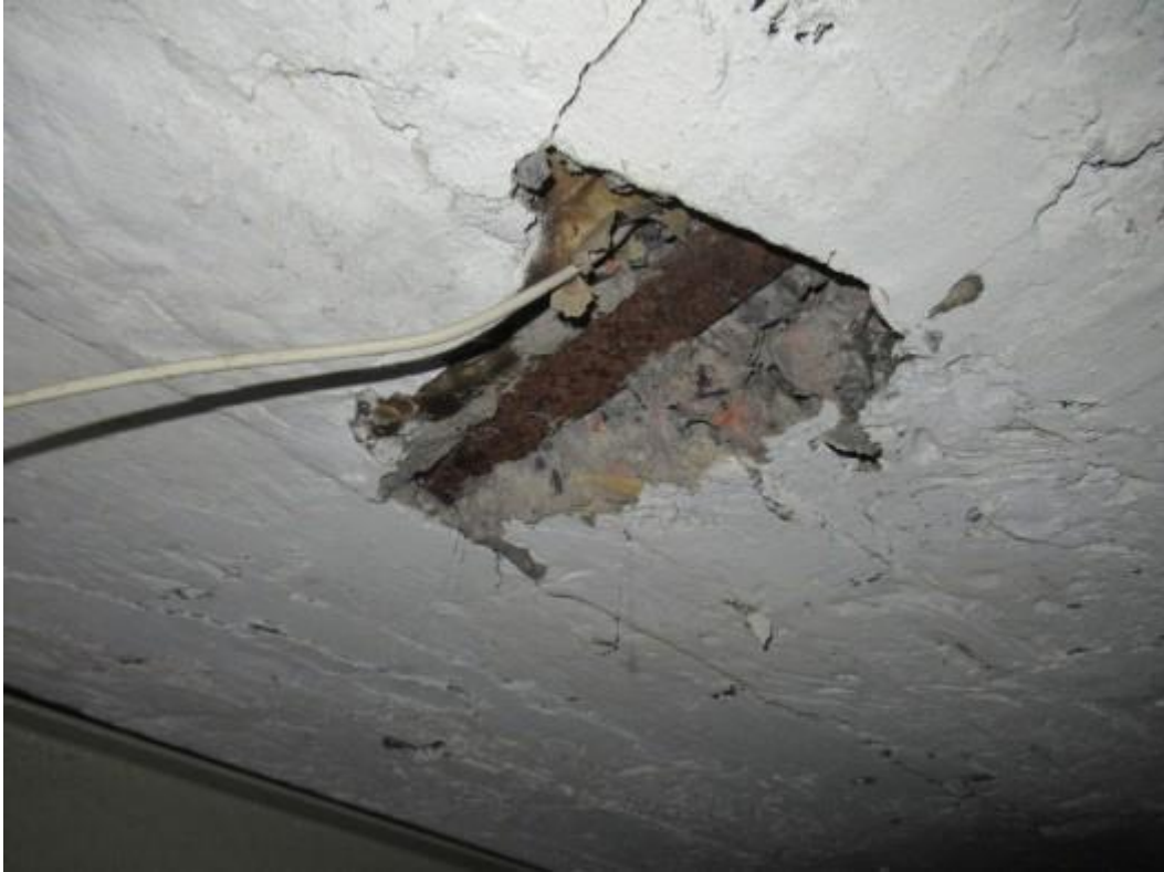
Typical condition of underside of reinforced concrete floor to the ground floor. The photograph shows spalling and damage of the concrete. This has exposed steelwork above with corrosion evident.
