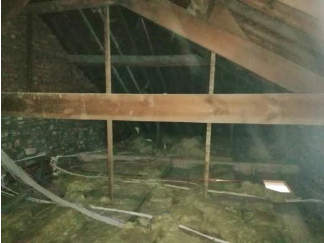
Roof void to the right hand side of the main building. This is to the main section of roof and not the lower level right hand side roof area. The photograph shows timber purlins and rafters.
