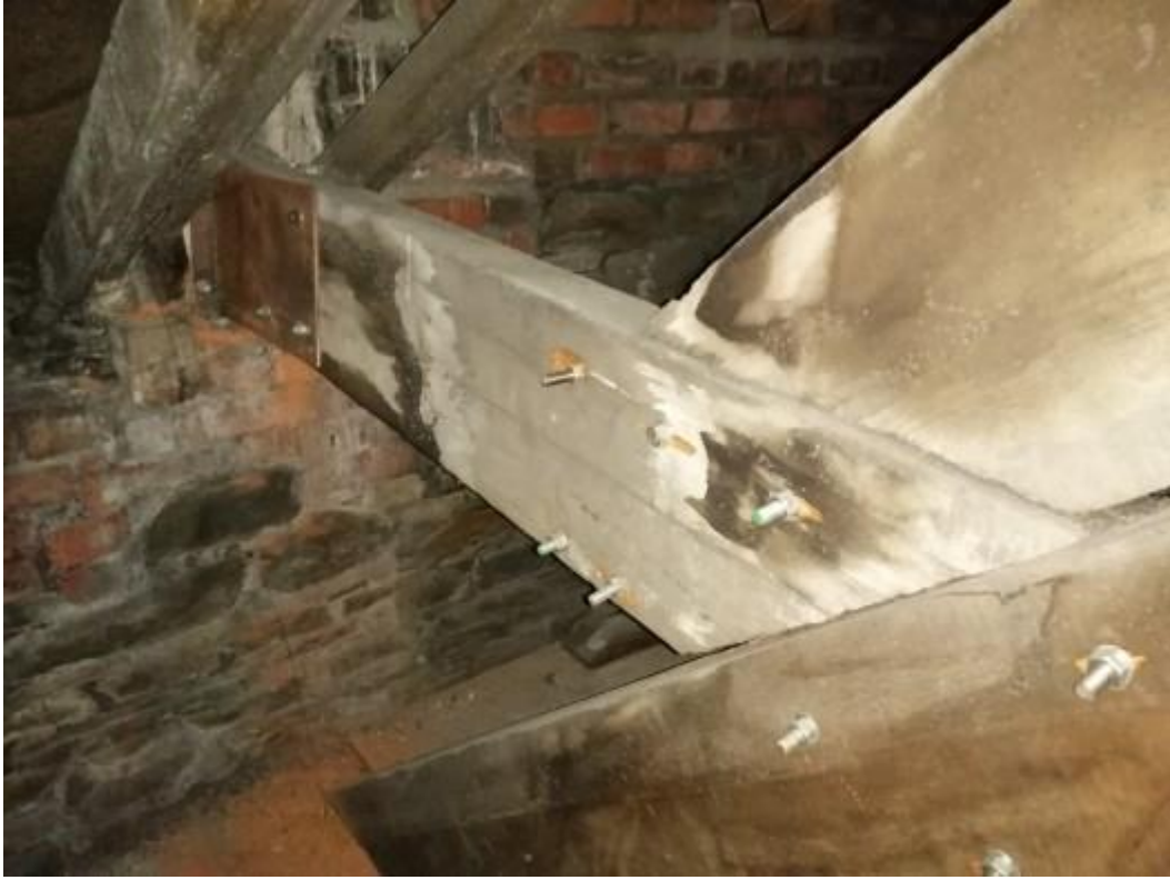
Further illustration of past repair where extending towards the front gable with additional steel plates provided.
