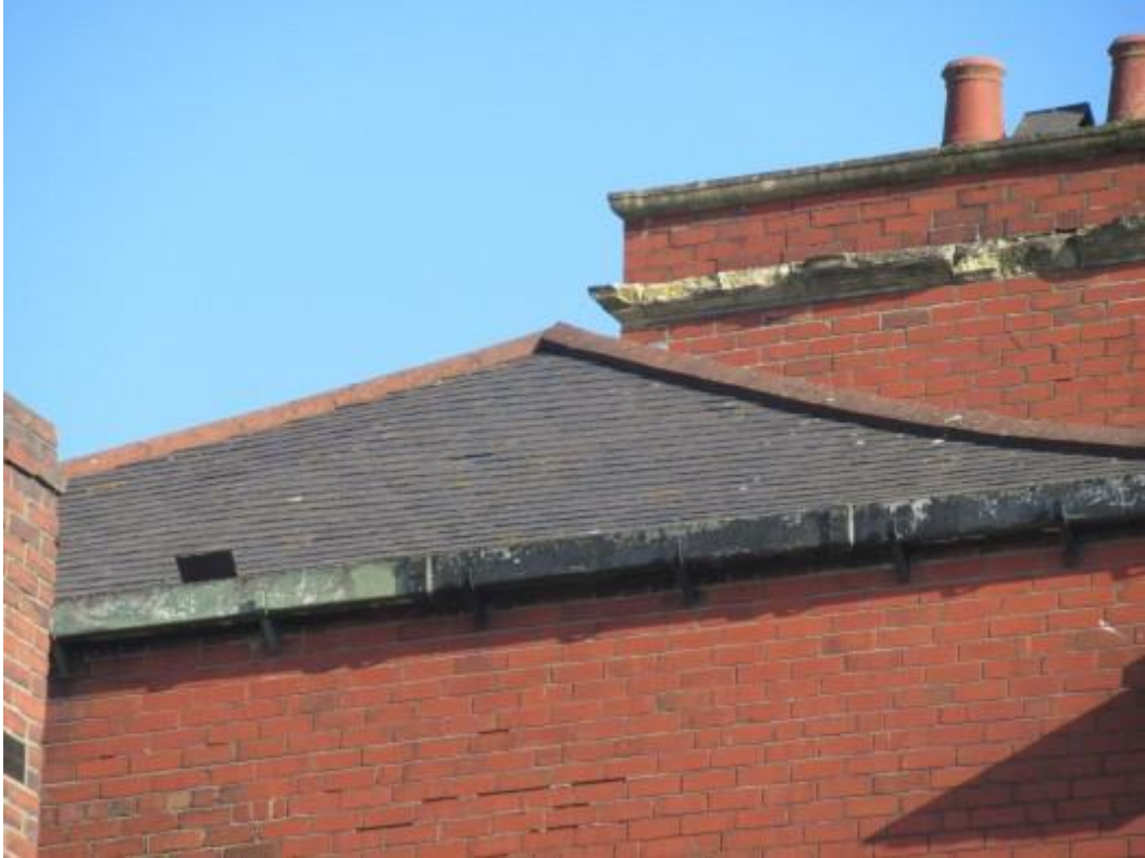
Further illustration of the left hand side roof slope with failed slates noted.
