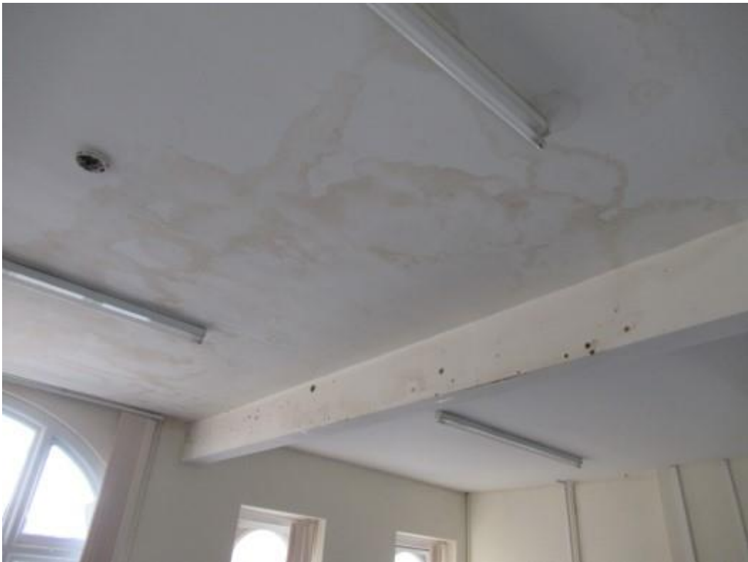
Further illustration of staining and damage to ceiling to upper floor accommodation. This is noted to the front section of the property where facing the front gable. Replacement work will be required.
