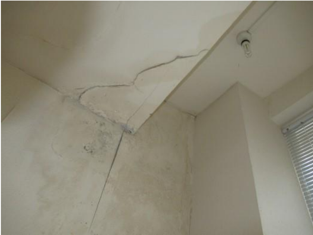
Further illustration of typical damp affected and damaged plaster finishes to the upper floor accommodation consistent with water ingress.
