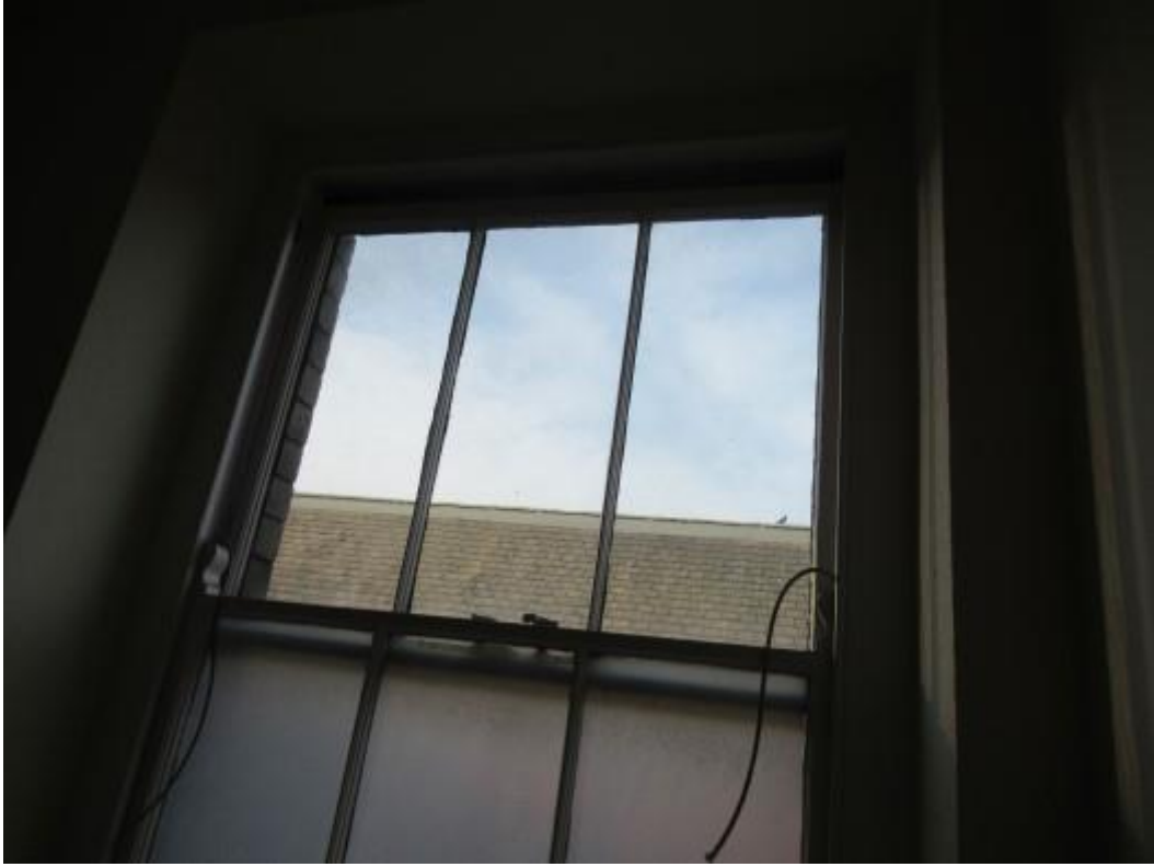
Typical failed sash cords to box sash window.
