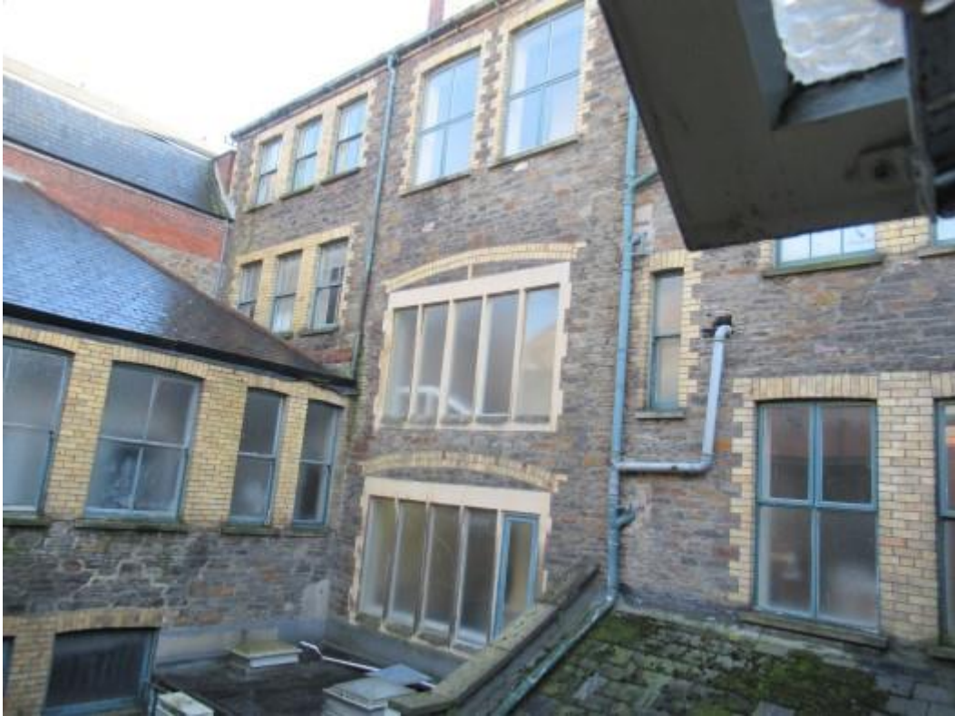
Windows to the rear of the main building. The windows comprise a mixture of box sash and softwood timber casement units. The windows will require overhauling and refurbishing as necessary.
