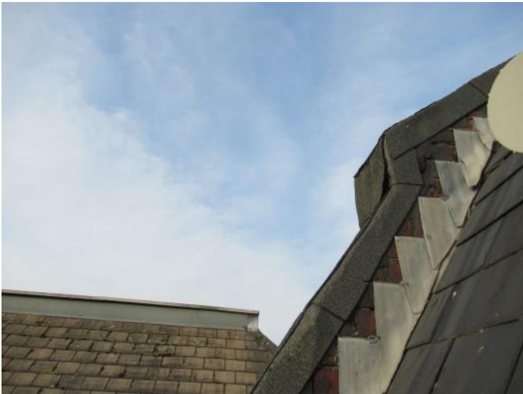
Further illustration of bitumen felt covering. This does not provide a satisfactory long term solution and upgrading works are required.
