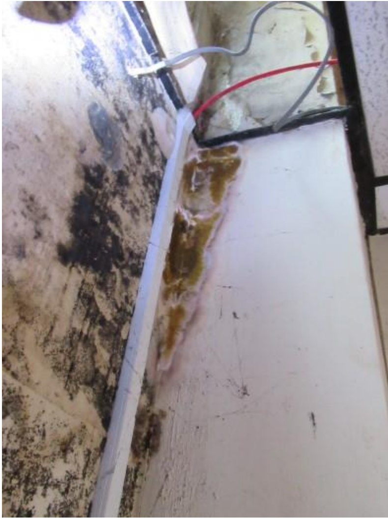
Further illustration of dry rot fungus to the rear.
