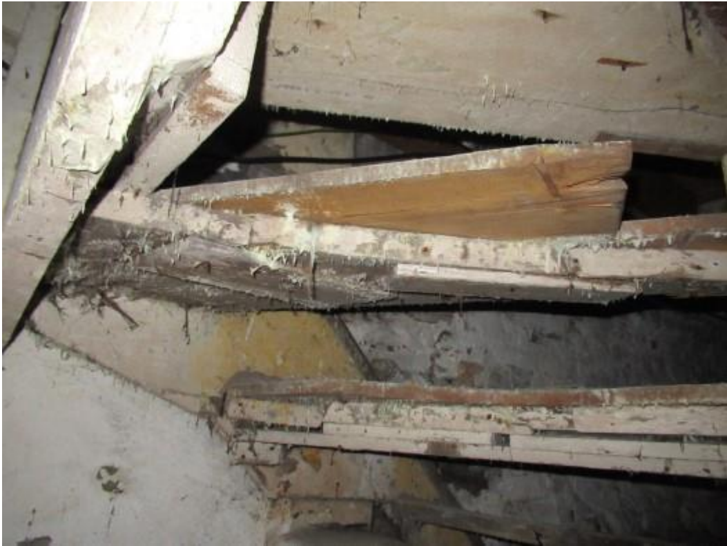
Fungal growth to underside of redundant timbers to the basement area. The timbers to this area will require removal. Timber treatment work will also be necessary.
