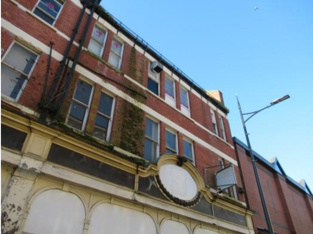
Further illustration of the right hand side elevation. The photograph shows deterioration of the brickwork consistent with leakage of rainwater goods. General staining and localised damage to the stone detailing is also noted.
