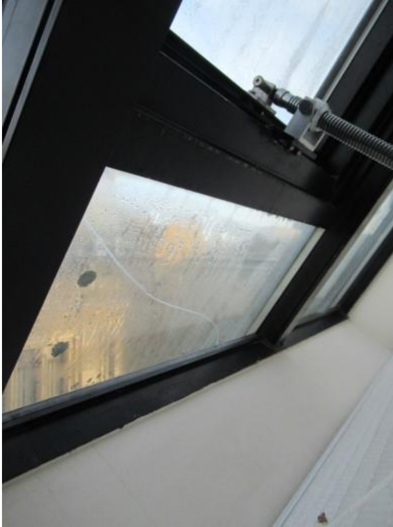
Further illustration of glazing to roof light with cracked glazing and condensation noted.
