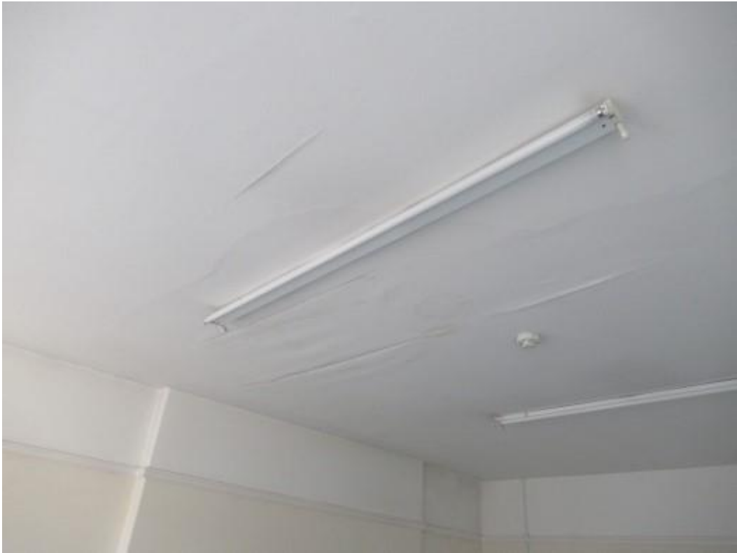
Typical cracking and deterioration of ceiling to upper floor accommodation.
