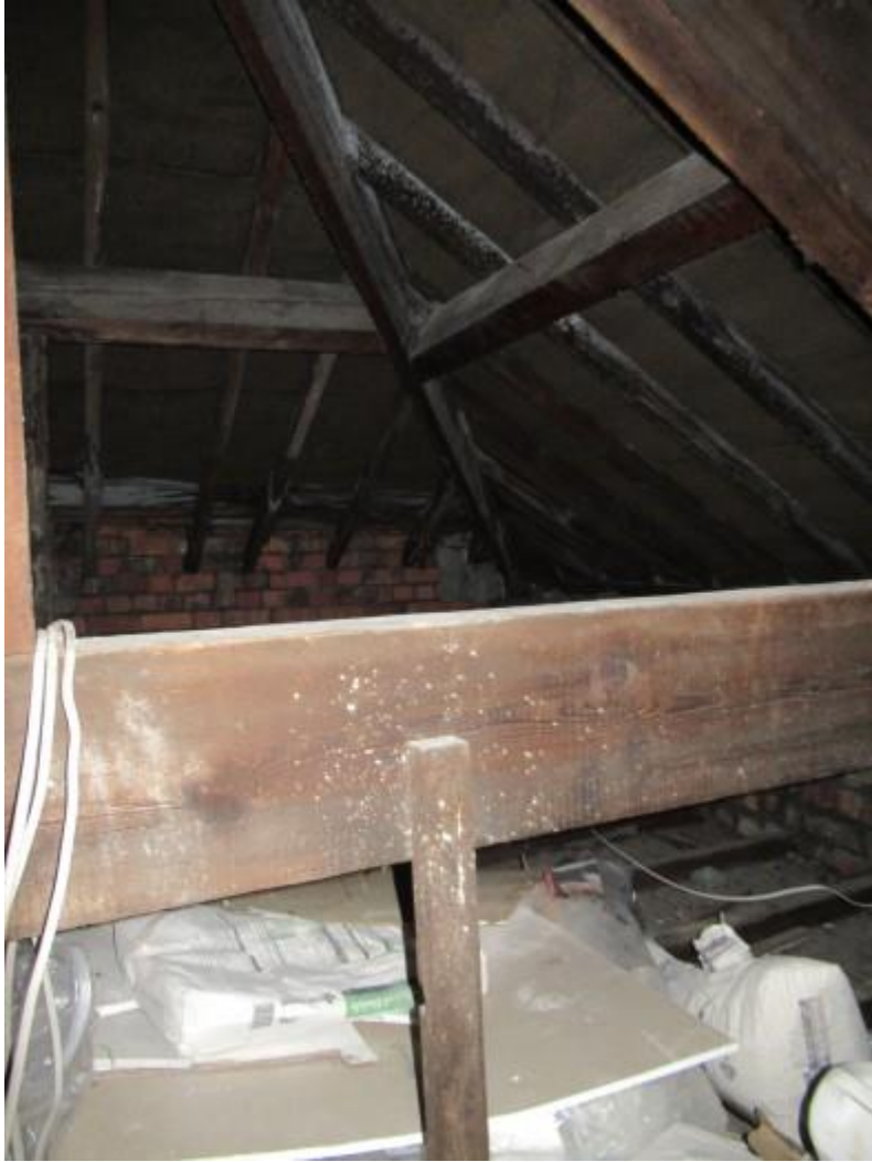
Further illustration of roof timbers to the right hand side lower level roof area. The photograph shows condensation staining to the underside of the timbers consistent with inadequate ventilation.
