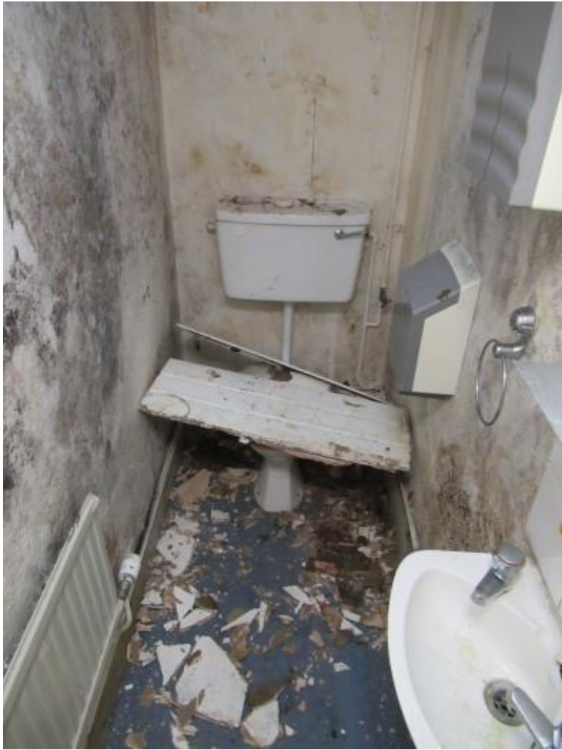
Poor condition of sanitary fittings to the rear of No. 80.
