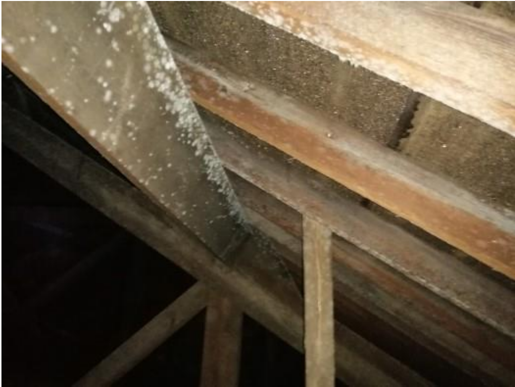
Typical moisture to underside of sarking felt and condensation to roof timbers.
