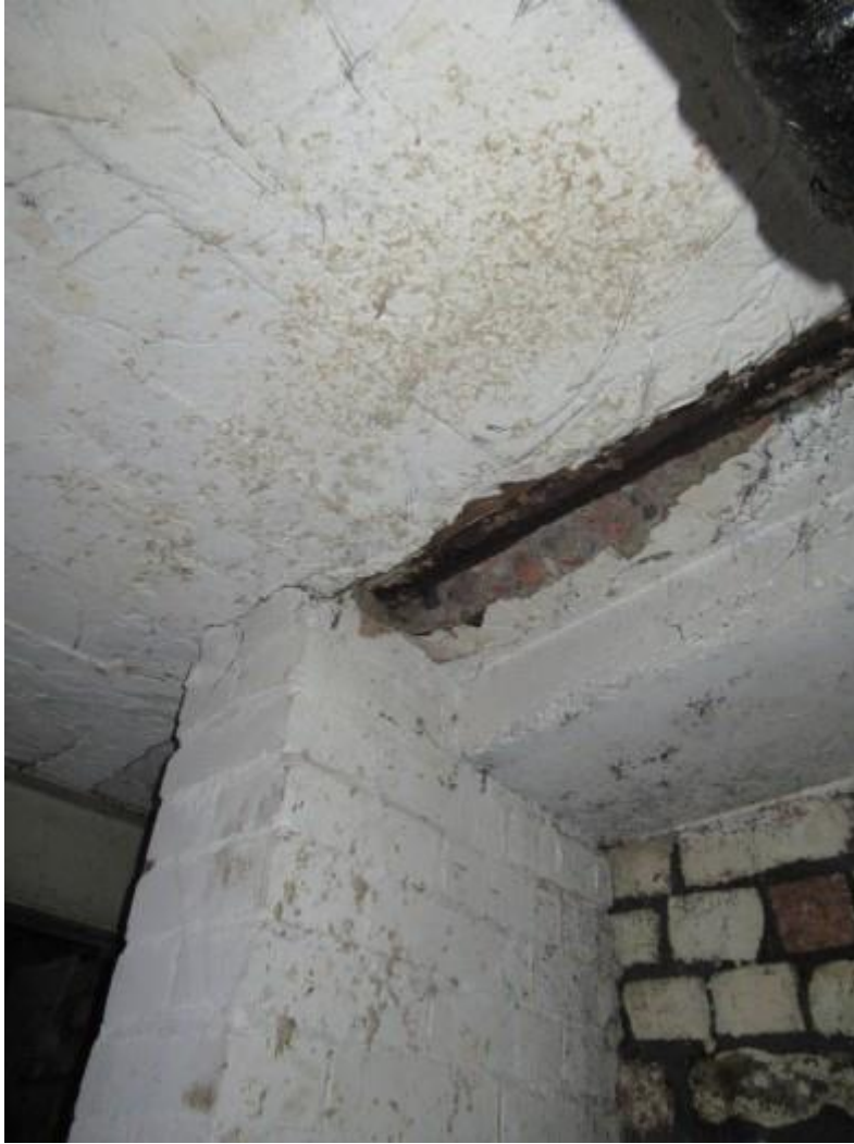
Further illustration of typical spalling and damage to underside of suspended concrete floor with corrosion noted.
