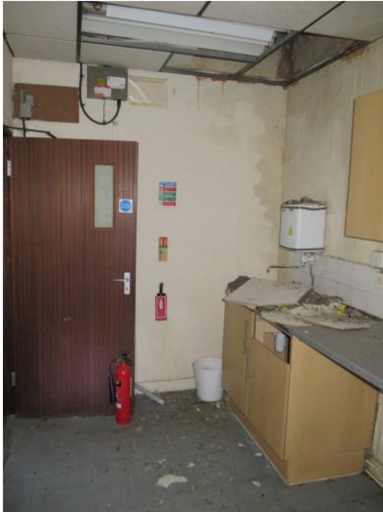
Poor condition of the kitchen units to the rear of the ground floor right hand side unit.
