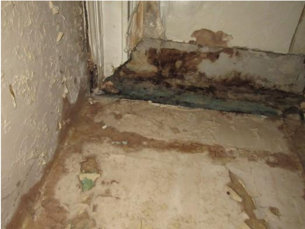
Dry rot above ceilings to the rear kitchen. There is further significant dry rot within the timbers where extending above this area.
