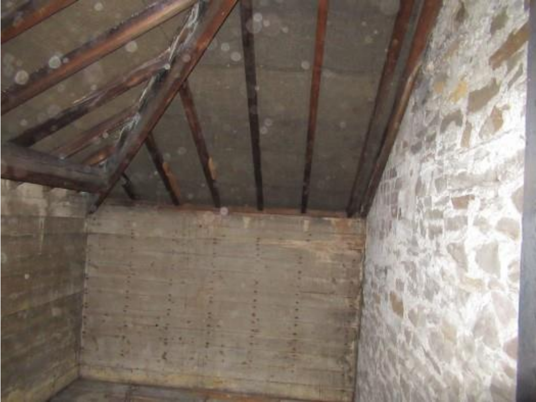
Further illustration of timbers to the right hand side of the roof. The photograph shows the principal hip rafter towards the front right hand corner of the roof. Staining of the timbers indicative of condensation is evident.
