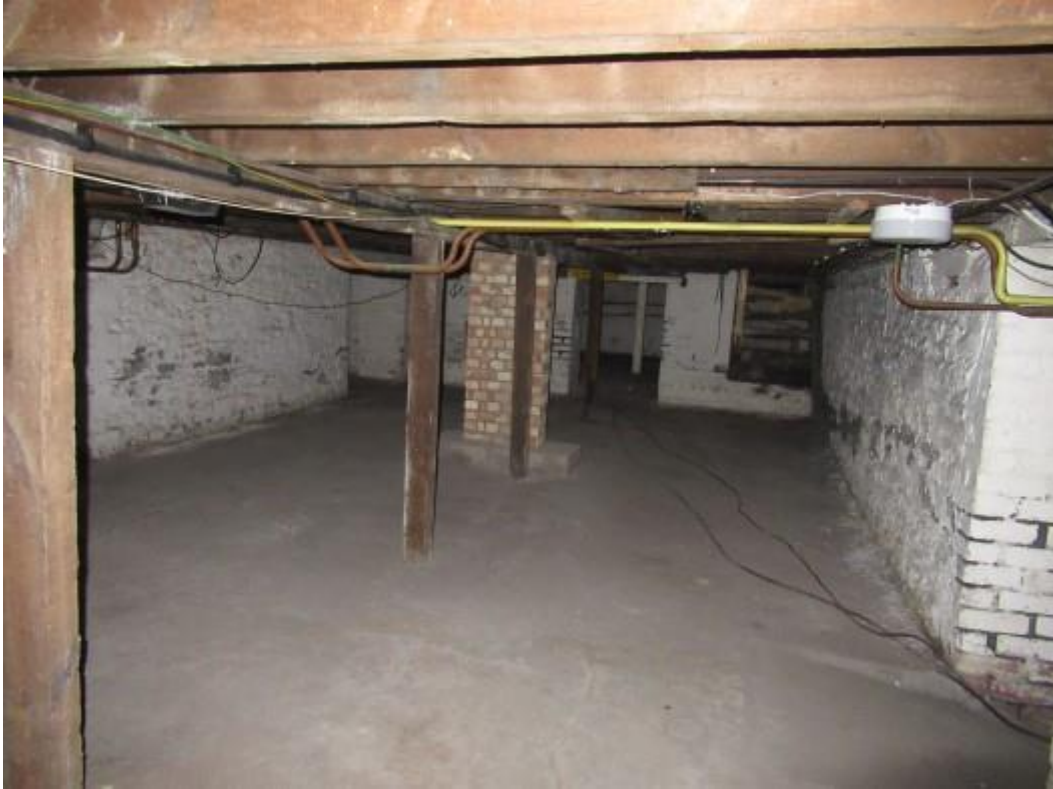
Further illustration of typical condition of underside of ground floor as viewed from the basement area. The photograph shows various intermediate supports to the flooring including brickwork pillars and timber struts to the underside of timber beams.
