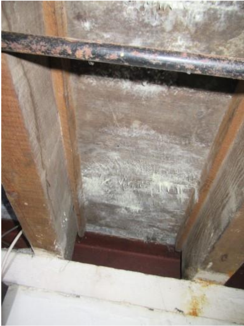
Fungal growth to the underside of timbers to the basement area.
