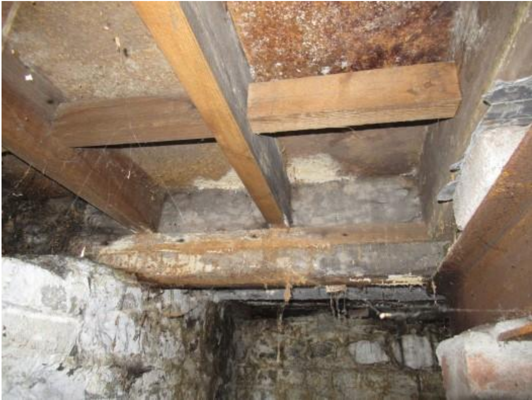
Further illustration of underside of timbers to the basement area with active wood boring insect infestation and fungal growth to timbers noted.
