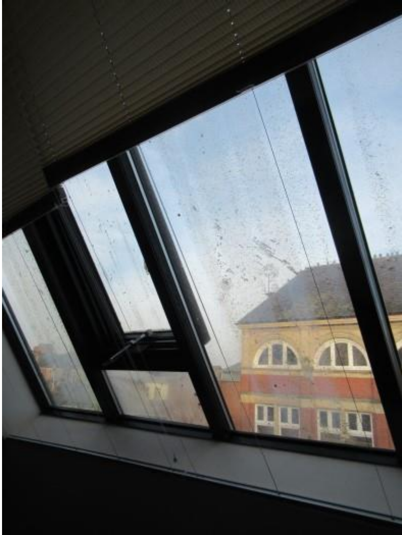
Internal view of roof lights to the right hand side elevation of the property. The photograph shows general staining and discolouration together with failed glazing. Interstitial condensation within double-glazing was noted.
