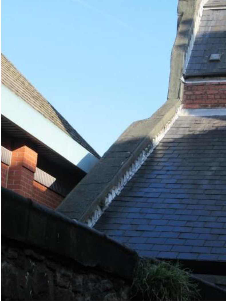
Further illustration of bitumen felt covering to rear parapet.
