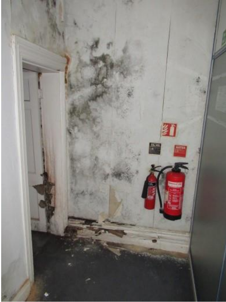
Damp affected and damaged plaster finishes to the rear of the first floor. The photograph also shows significant dry rot.
