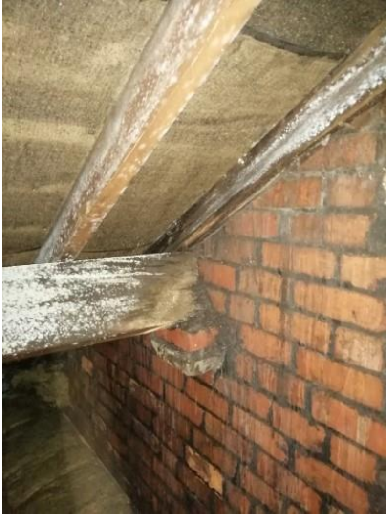
Further illustration of condensation to underside of roof timbers to the central roof area.
