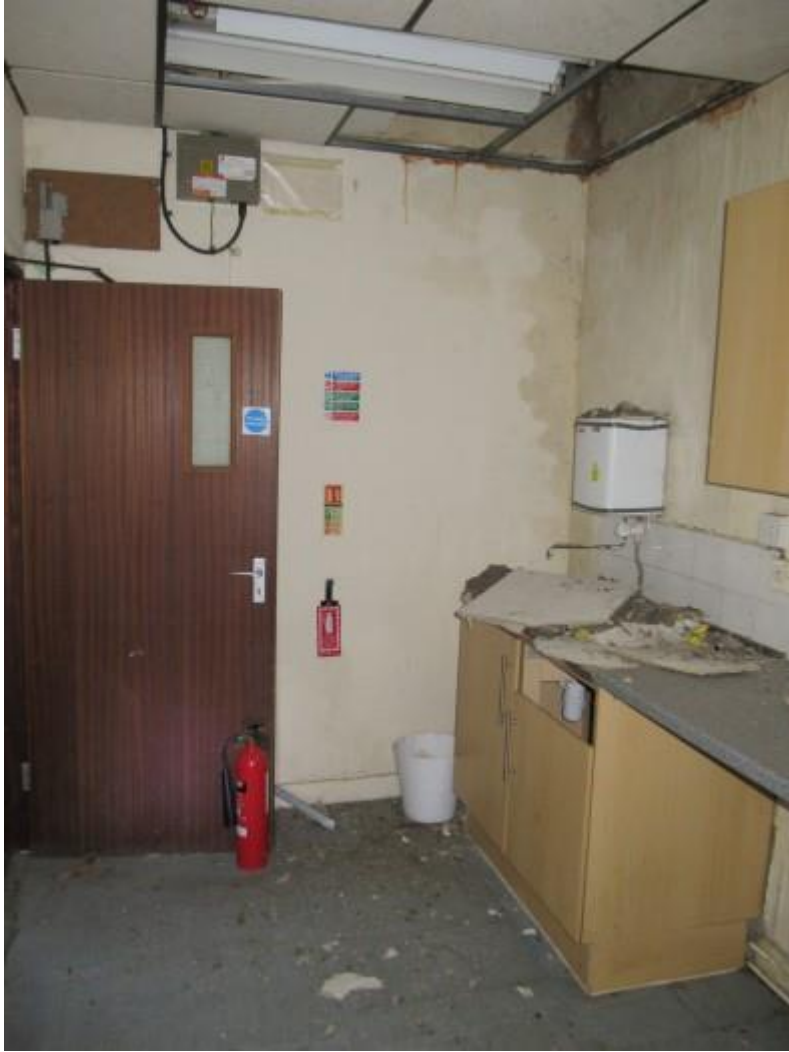
Kitchen area serving the ground floor right hand side unit with water ingress noted. There is significant dry rot to this area. The water ingress is consistent with deterioration of flashings and roof coverings above.
