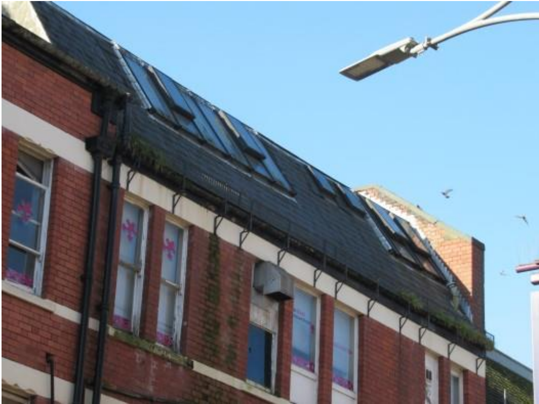
Guttering to the right hand side of the property. The photograph shows extensive vegetation and leakage. This is contributing to internal damp.
