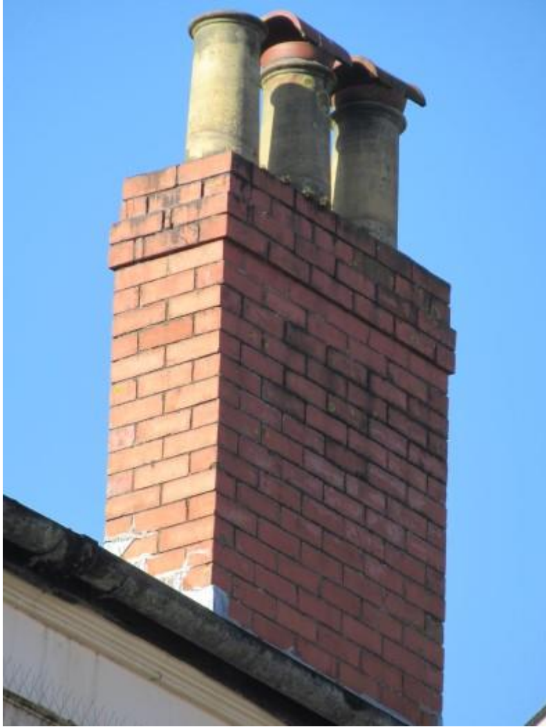
Chimney stack to the right hand side of the property. There is significant water ingress at the base of the chimney stacks to the right hand side of the property.
