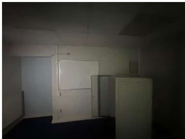
Figure 4 Basement wall for proposed removal (4)
