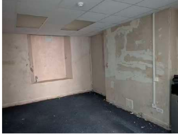
14. Basement room; loss of window and fireplace
