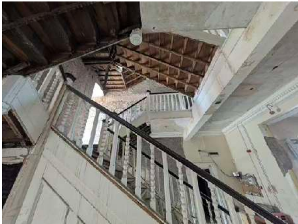
4. View of staircase and extent of water damage
