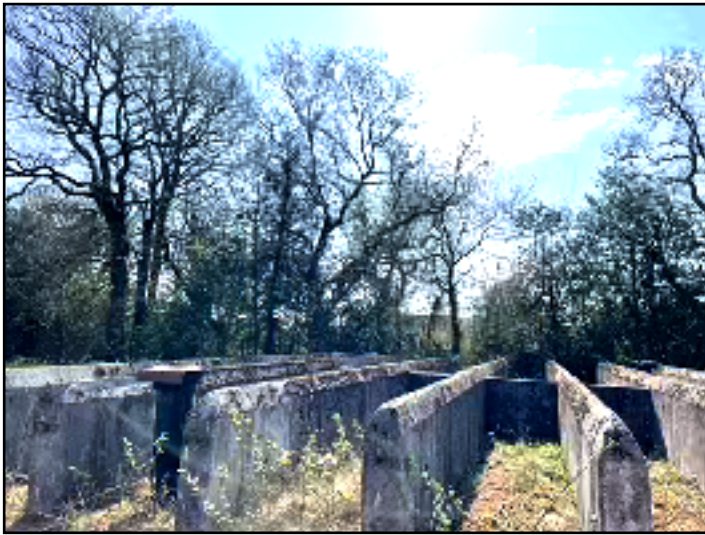
Photo 9. Concrete slabs with moss and bramble growth along hardstanding.
