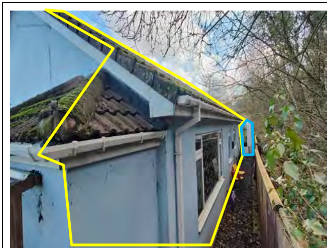
Photo 5. The southwestern elevation of the day centre main building (yellow) and northwestern elevation of the conservatory (blue).
