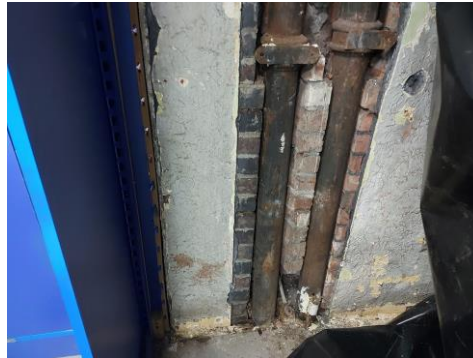
Figure 8- Existing soil pipes - see plan
