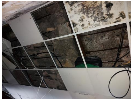
Figure 1- Underside of Patio / Reinforced Concrete slab
