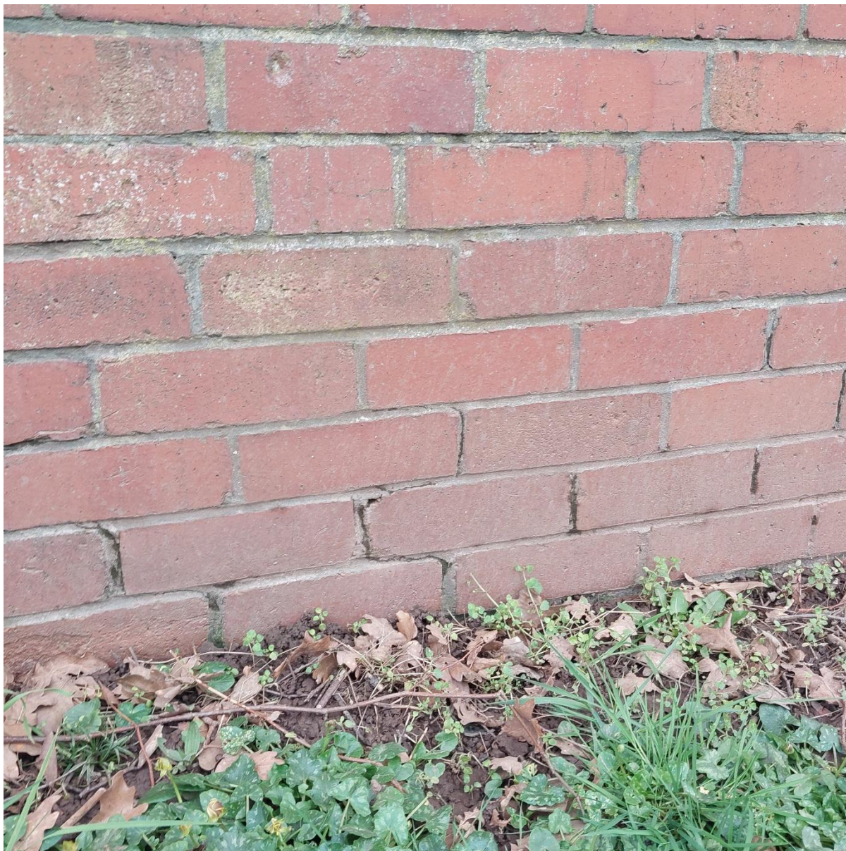
Picture 5 – cracks evident in the wall
