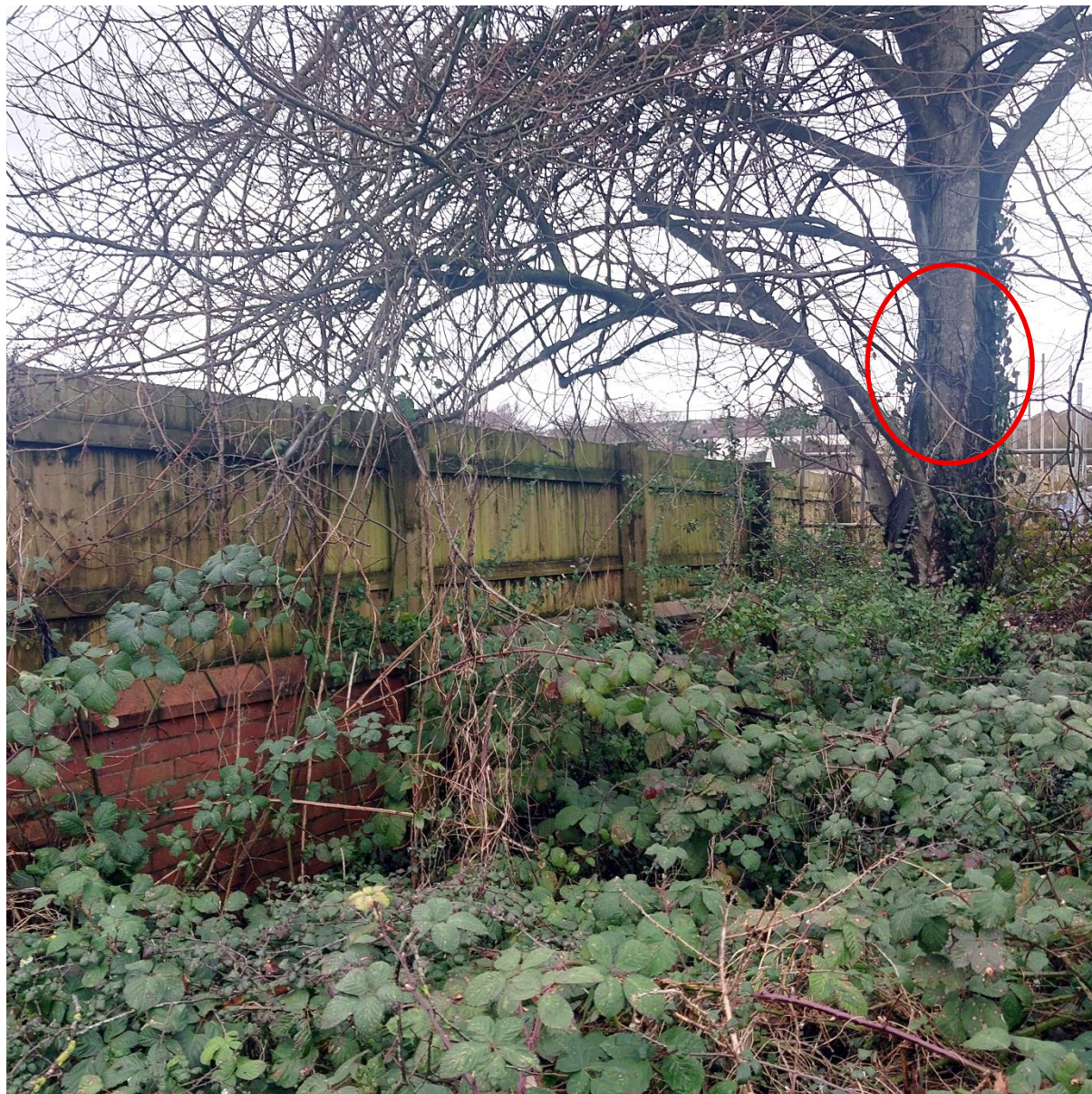
Picture 6 – relationship of tree and boundary wall. red circle overlays the compression defect.
