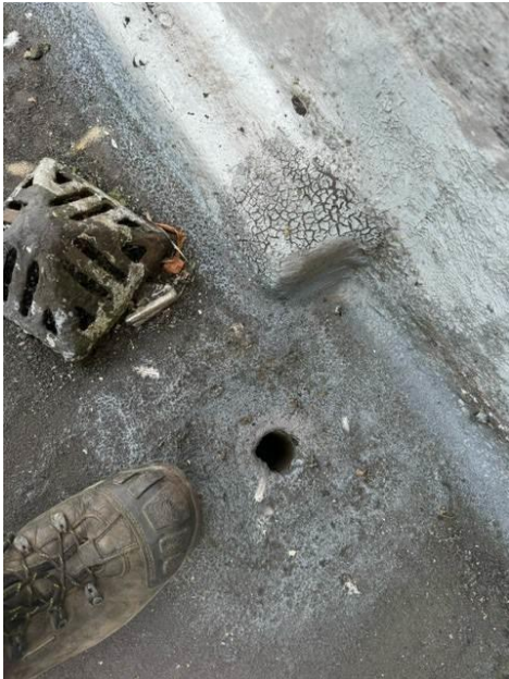
Left: typical view of a 'sleeved' outlet
