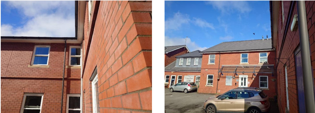
Figure 4-2: Steel ducting running the length of the building.
