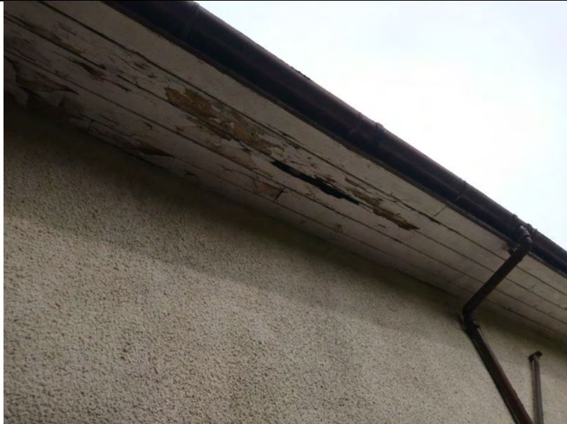
Hole in soffit approx. 3-4cm across by 40cm long – broken panel
