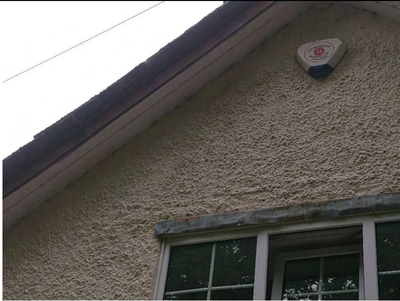
Very small gap between soffit and wall
