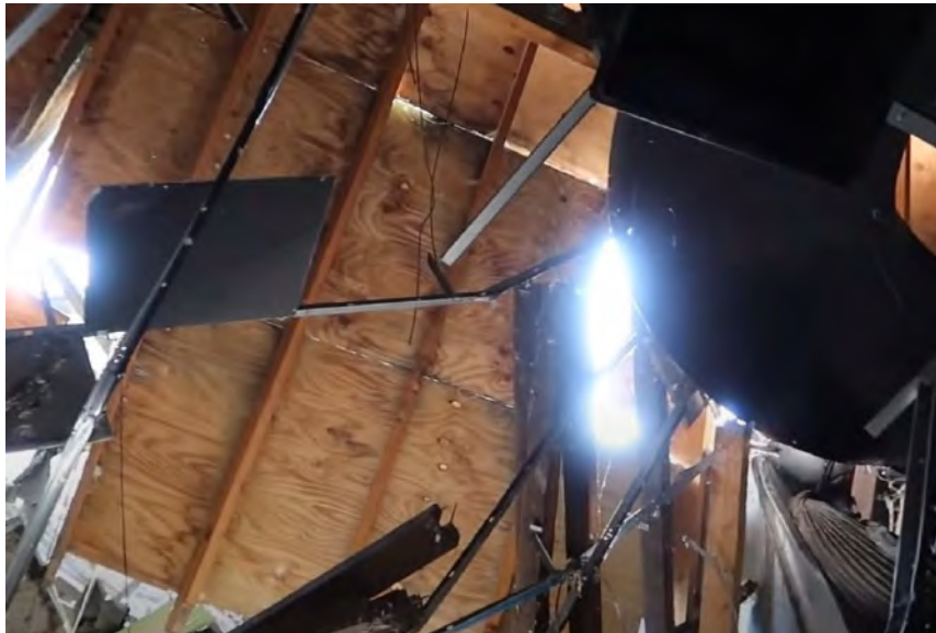
Figure A43. Image of part of the failing roof structure prior to the 2018 fire taken from https://www.youtube.com/watch?v=QVJ7g2Xw1Hg
