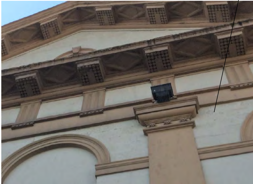
Figure A33. Apparent differing areas of stonework detailing beneath the paint
