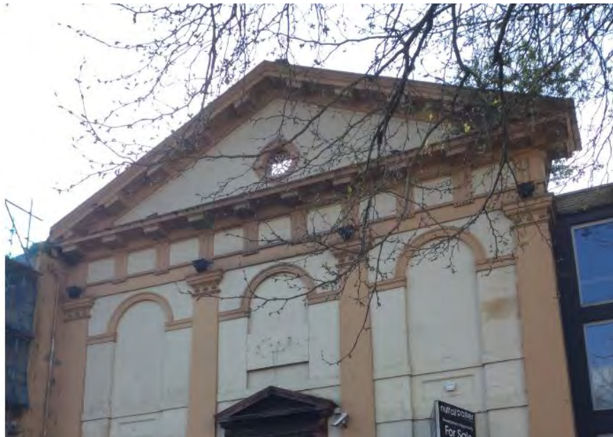
Figure A67. The pediment after the fire with the finials no longer apparent
