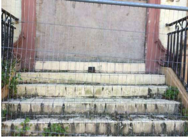
Figure A34. Original step finishes lost. Steps covered in slip resistant, modern tiles.
