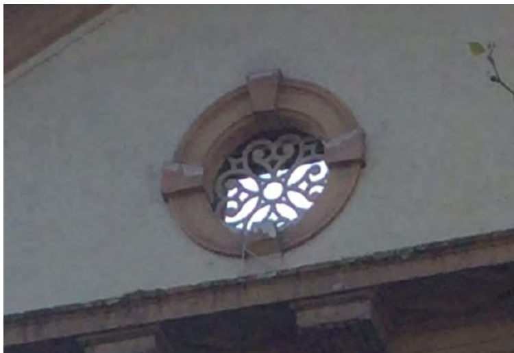
Figure A36. Ornate iron ventilation grill within the pediment oculus with damaged stone surround
