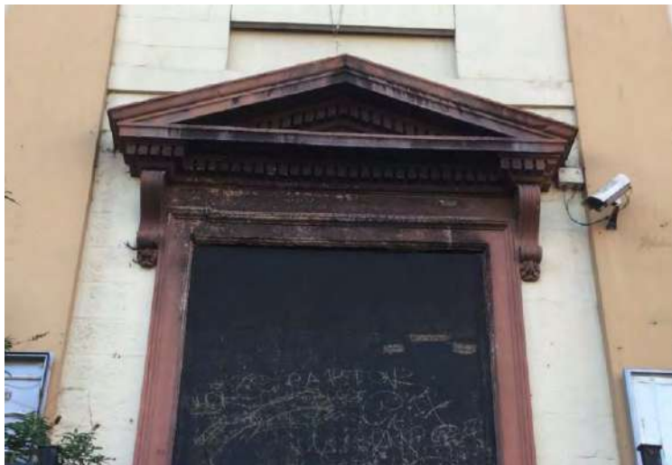
Figure A35. Doorcase in poor condition. Boarding over the door concealing the entrance and possible doors.
