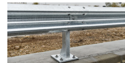
Galvanised steel Armco vehicle barrier to protect fencing adjacent to vehicle circulation routes.
