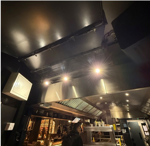
EXISTING DUCTWORK AND CANOPY POSITION IN KITCHEN AREA BELOW
