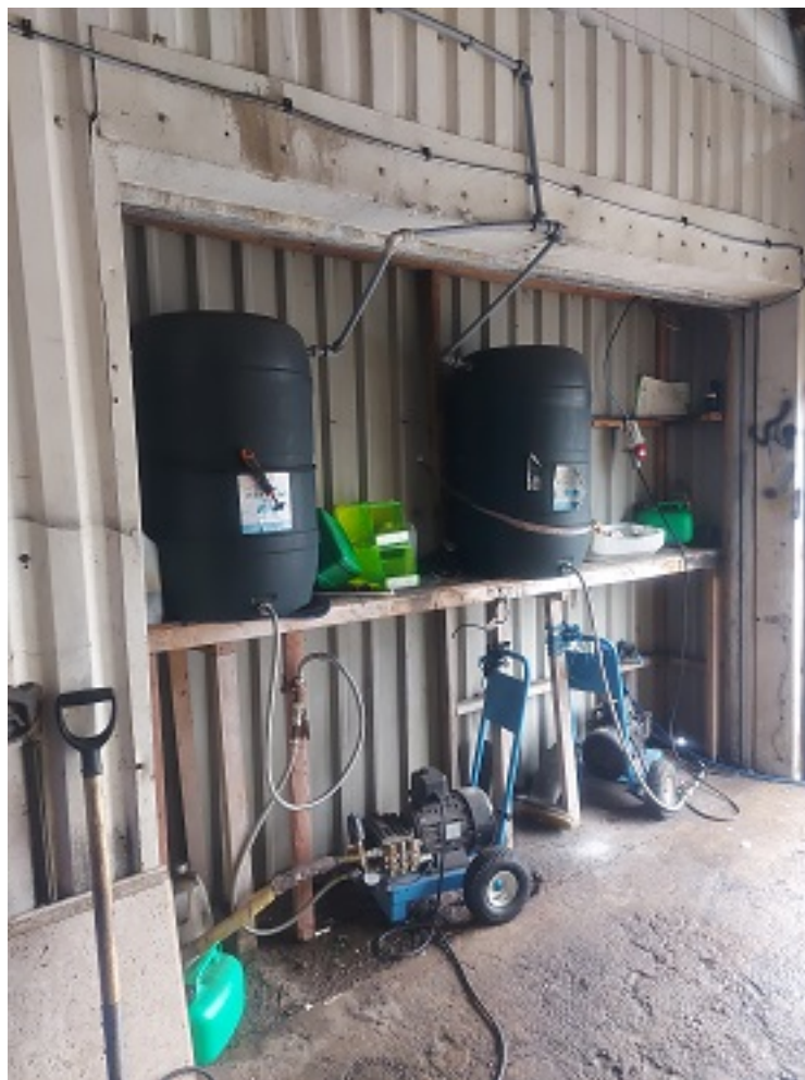
Image 19: 19. Garage water connections
