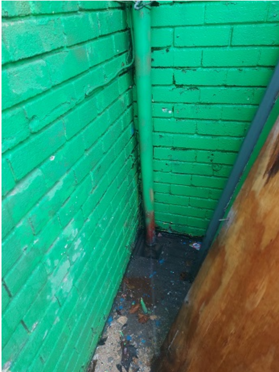
Image 10: 10. Garage / Store front - drainage gulley
