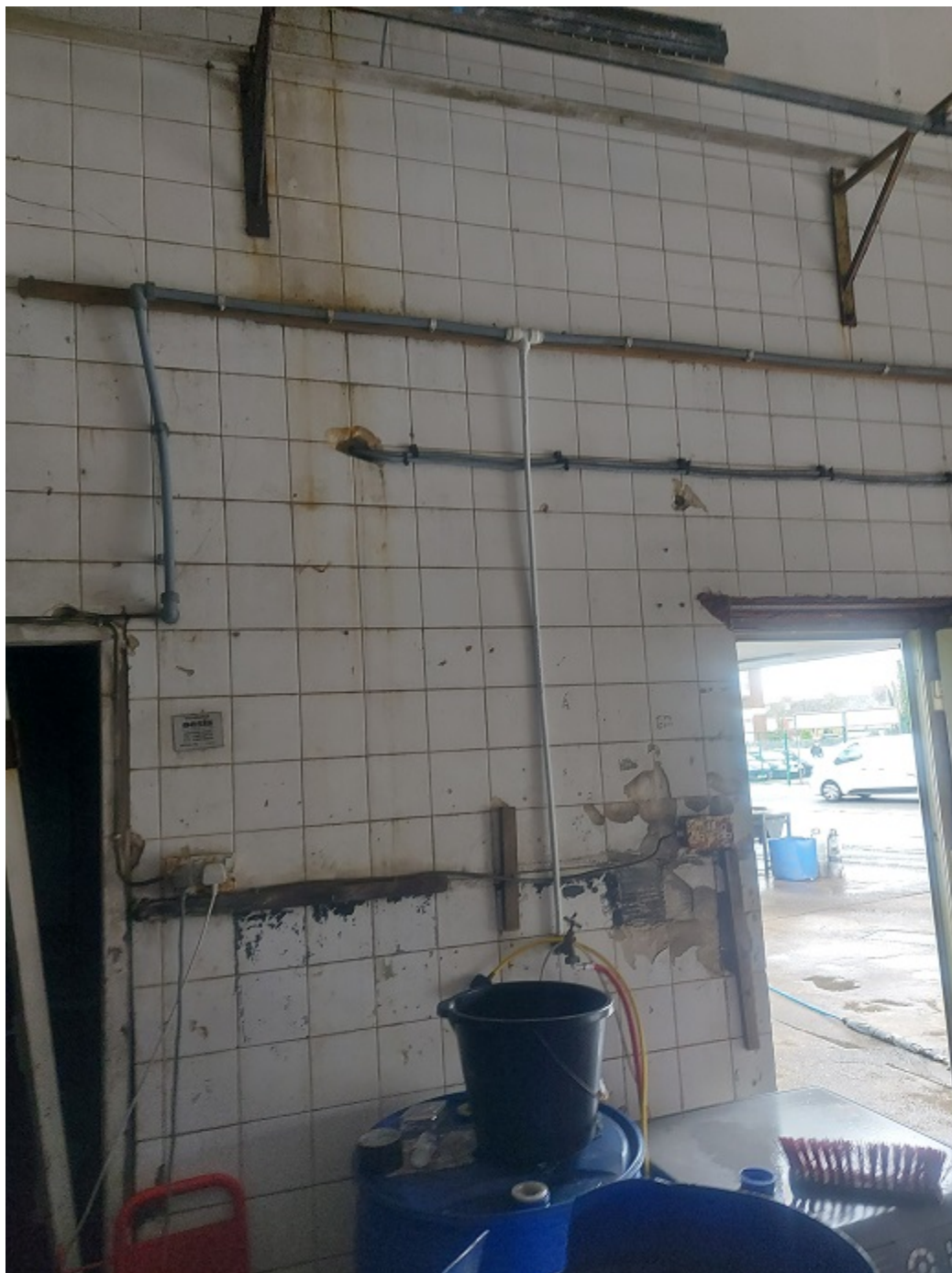
Image 17: 17. Garage water supply lines
