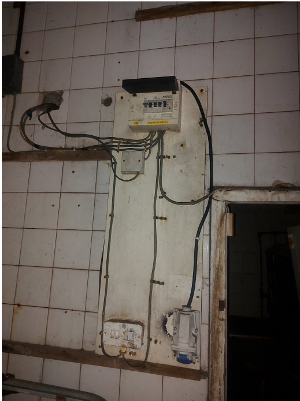
Image 18: 18. Garage electrical supplies
