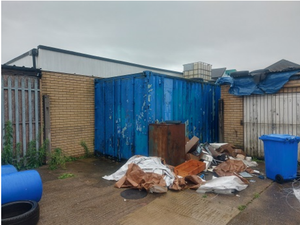
Image 4: 4. Rear Elevation showing trade waste & container
