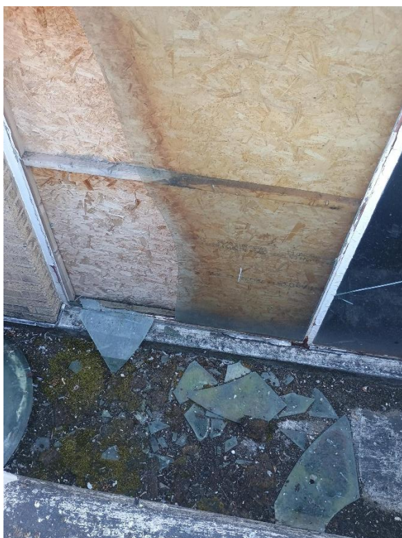
Left: image showing extent of deterioration to Lantern Room windows.
