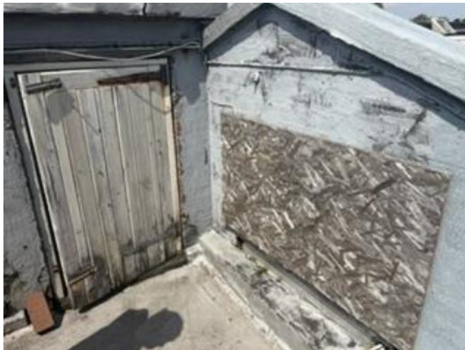
Left: image showing typical condition of service duct doors and frames.
