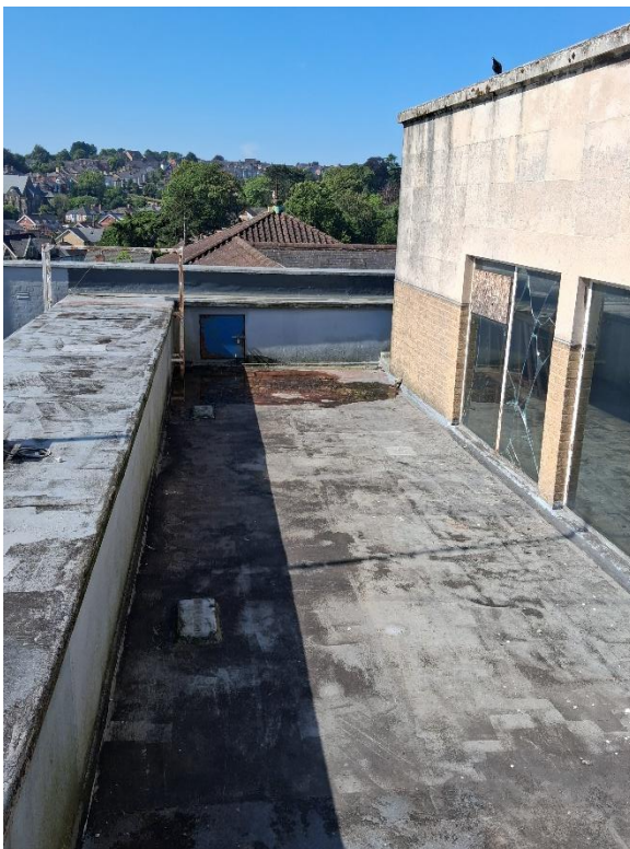
Left: view of roof with inadequate falls and drainage.
