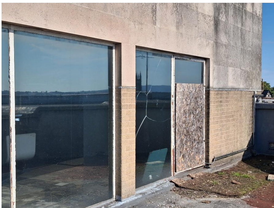
Left: typical view of existing condition of Lantern Room windows.
