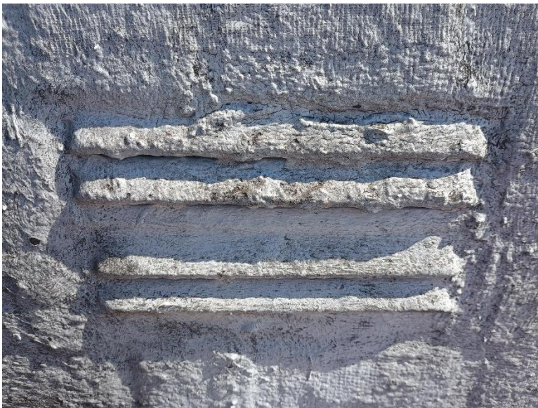
Left: typical image of existing cavity vents blocked by waterproof coatings.
