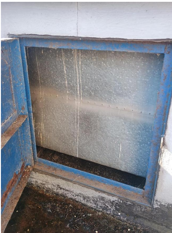
Left: internal view of redundant door to air-handling ductwork.
