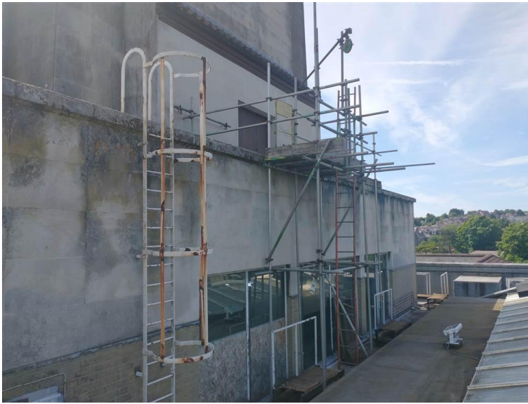
Left: existing badly corroded cat ladder.
