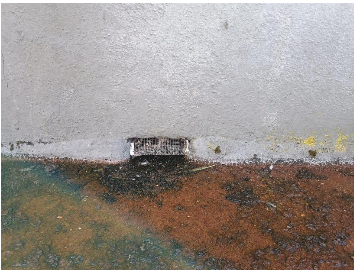
Left: image of the existing sub-standard drainage arrangement.
