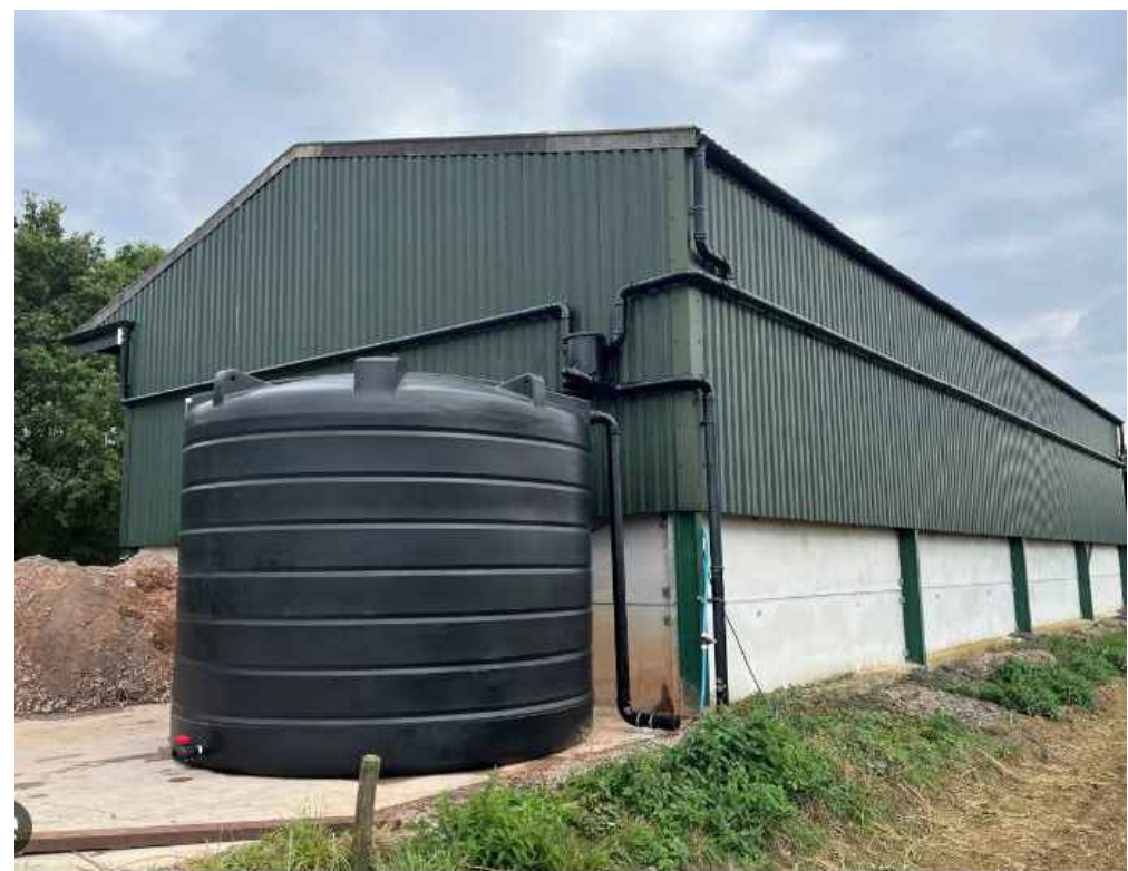
Rain Water harvesting tank with filter.
