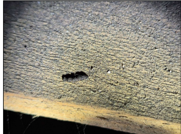
Figure 23 – Bat Dropping on Timber Stored within Builder's Bag in Shed 3
