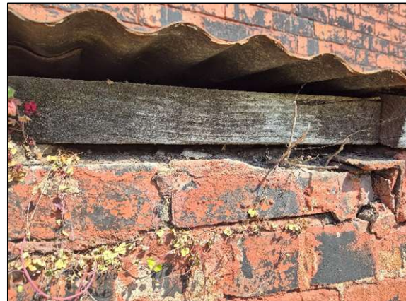
Figure 15 – Gap beneath Corrugated Roof Sheets on Lean-to May Permit Access/Egress for Bats to Interior
