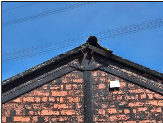
Figure 14 – Gap beneath Ridge Tiles on Gable Roof May Permit Access to Loft
