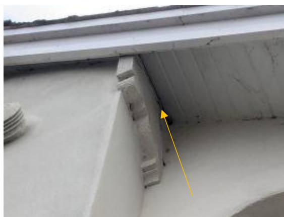
PRFs – Cavity in soffit – access to a cavity of unknown proportions, including bitumen membrane.
