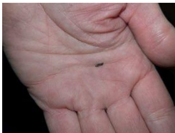
Pipistrelle type droppings identified in roof space.
