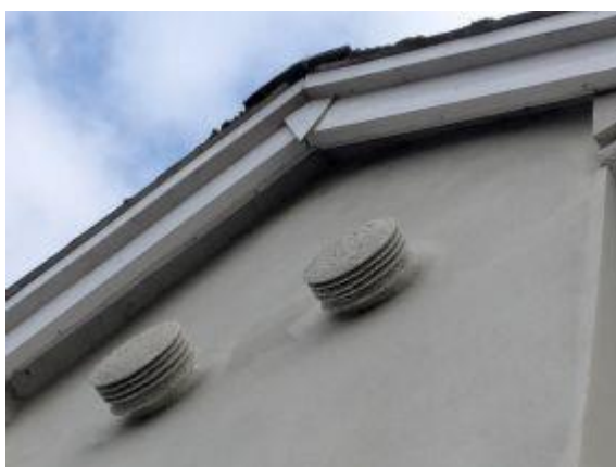
Soffits and bargeboards are mostly sealed
