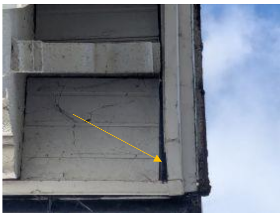
PRFs – Cavity in soffit – access to a cavity of unknown proportions, including bitumen membrane.
