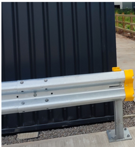
External Armco Safety Barrier Finish: Galvanised steel with end caps and fish tails where required
