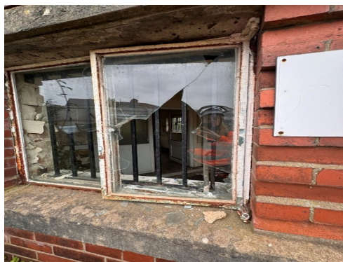
Photograph 4: u1b5-2 Broken window, entry point into the building.
