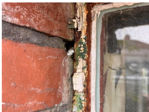
Photograph 6: u1b5-2 Missing mortar, external.
