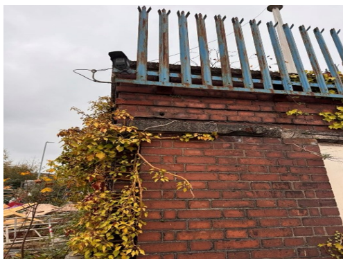
Photograph 3: u1b5-1 Hole within a brick wall.
