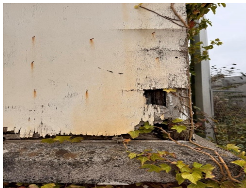
Photograph 2: u1b5-1 Hole within a window board.
