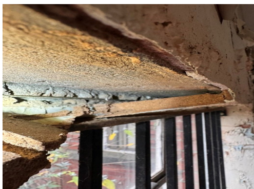
Photograph 5: u1b5-2 Damaged masonry, building interior.
