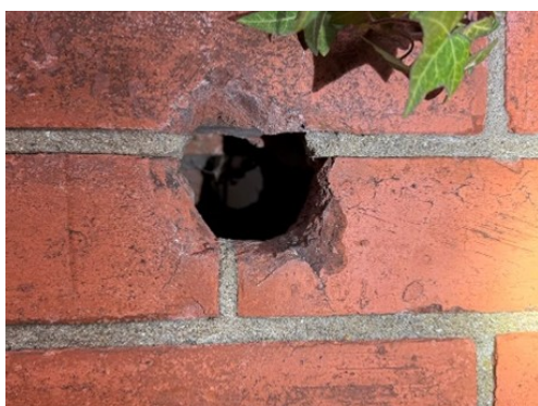
Photograph 7: u1b5-2 Hole within brickwork
