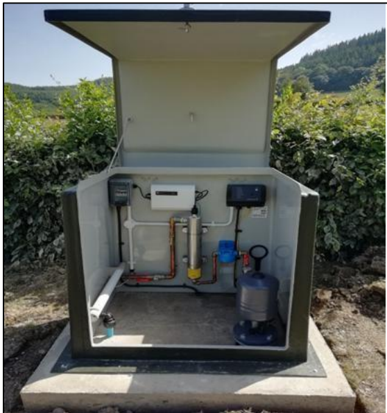
Photograph of an example GRP borehole installation.
