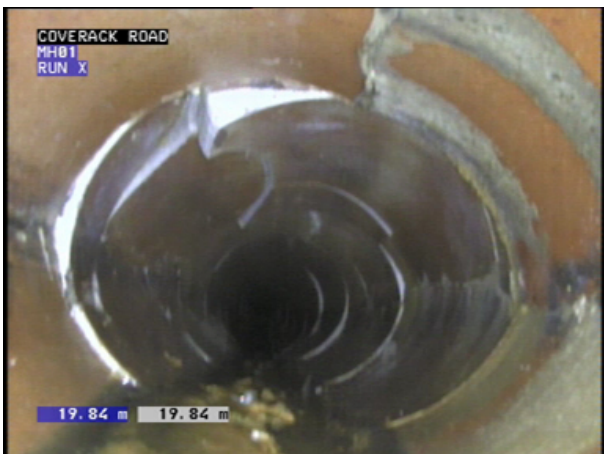
Photo: 3_3_46_A.jpg, 00:01:21 19.84m, Broken pipe, from 8 to 1 o'clock
