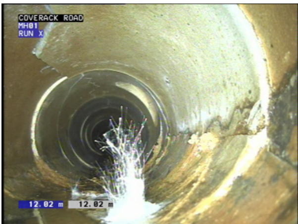
Photo: 3_3_32_A.jpg, 00:00:44 12.02m, Broken pipe, from 10 to 11 o'clock
