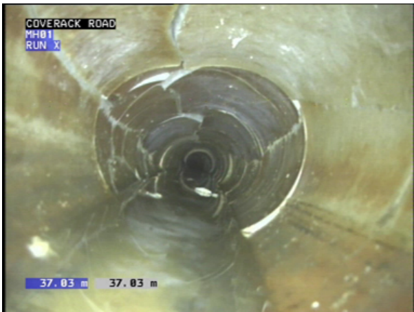
Photo: 3_3_79_A.jpg, 00:03:39 37.02m, Broken pipe, from 10 to 11 o'clock, Start
