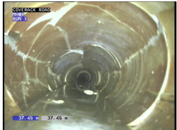
Photo: 3_3_81_A.jpg, 00:03:46 37.42m, Broken pipe, from 9 to 12 o'clock, Start
