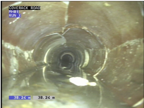
Photo: 3_3_84_A.jpg, 00:03:49 38.22m, Broken pipe, from 10 to 12 o'clock, Start
