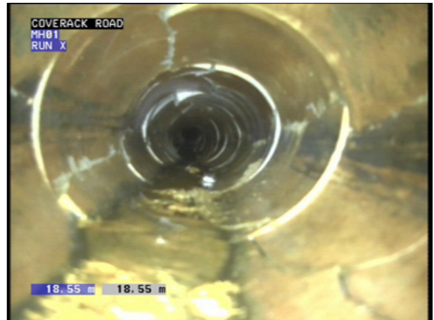
Photo: 3_3_43_A.jpg, 00:01:14 18.52m, Broken pipe, from 11 to 12 o'clock, Start
