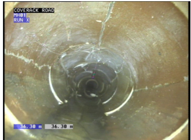
Photo: 3_3_78_A.jpg, 00:03:35 36.28m, Cracks, multiple, from 12 to 12 o'clock, Start
