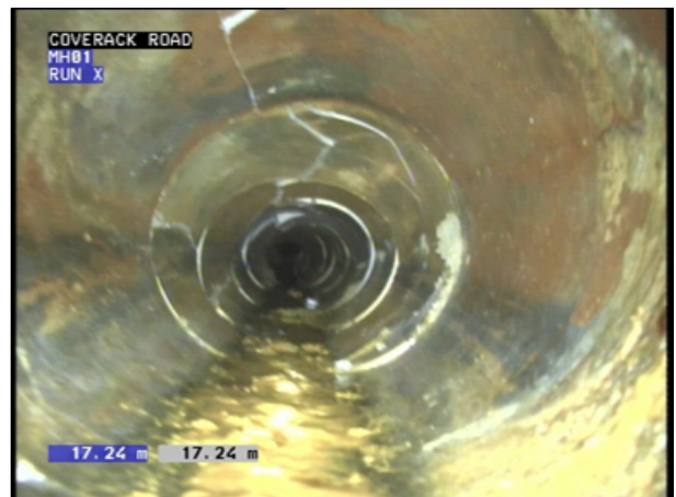
Photo: 3_3_41_A.jpg, 00:01:07 17.16m, Broken pipe, from 11 to 1 o'clock
