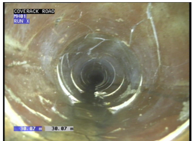
Photo: 3_3_63_A.jpg, 00:02:51 30.07m, Fracture, multiple, from 12 to 12 o'clock, Start
