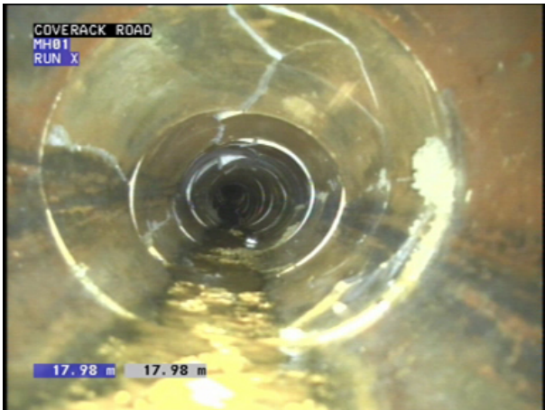
Photo: 3_3_42_A.jpg, 00:01:07 17.8m, Fracture, multiple, from 12 to 12 o'clock, Start
