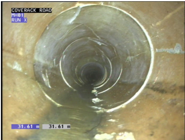
Photo: 3_3_69_A.jpg, 00:03:03 31.6m, Broken pipe at joint, from 11 to 12 o'clock
