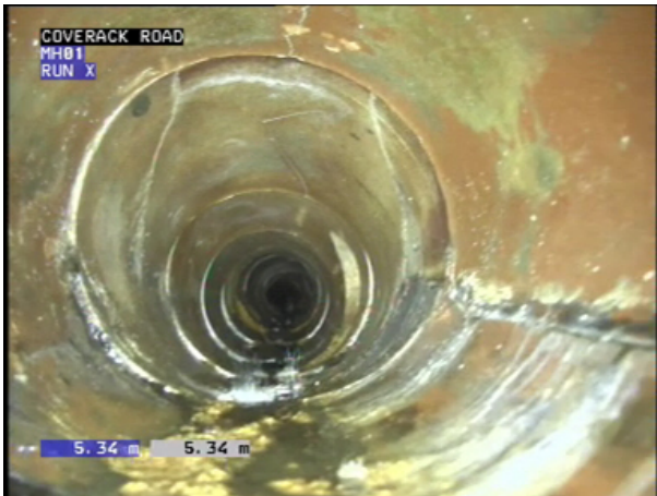
Photo: 3_3_19_A.jpg, 00:00:20 5.32m, Fracture, longitudinal, at 3 o'clock, Start
