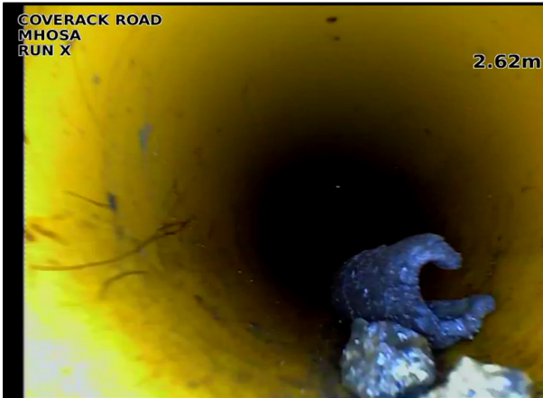
Photo: 7_7_142_A.jpg, 00:00:06 2.62m, Settled deposits, coarse, 20% cross-sectional area loss
