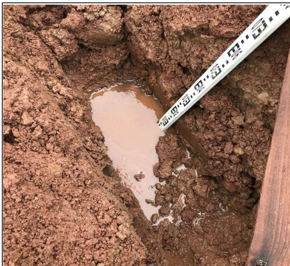
Plot 156 Membrane Placement (Membrane Placement Confirmed by Hand Touch Through Water Ingress)
