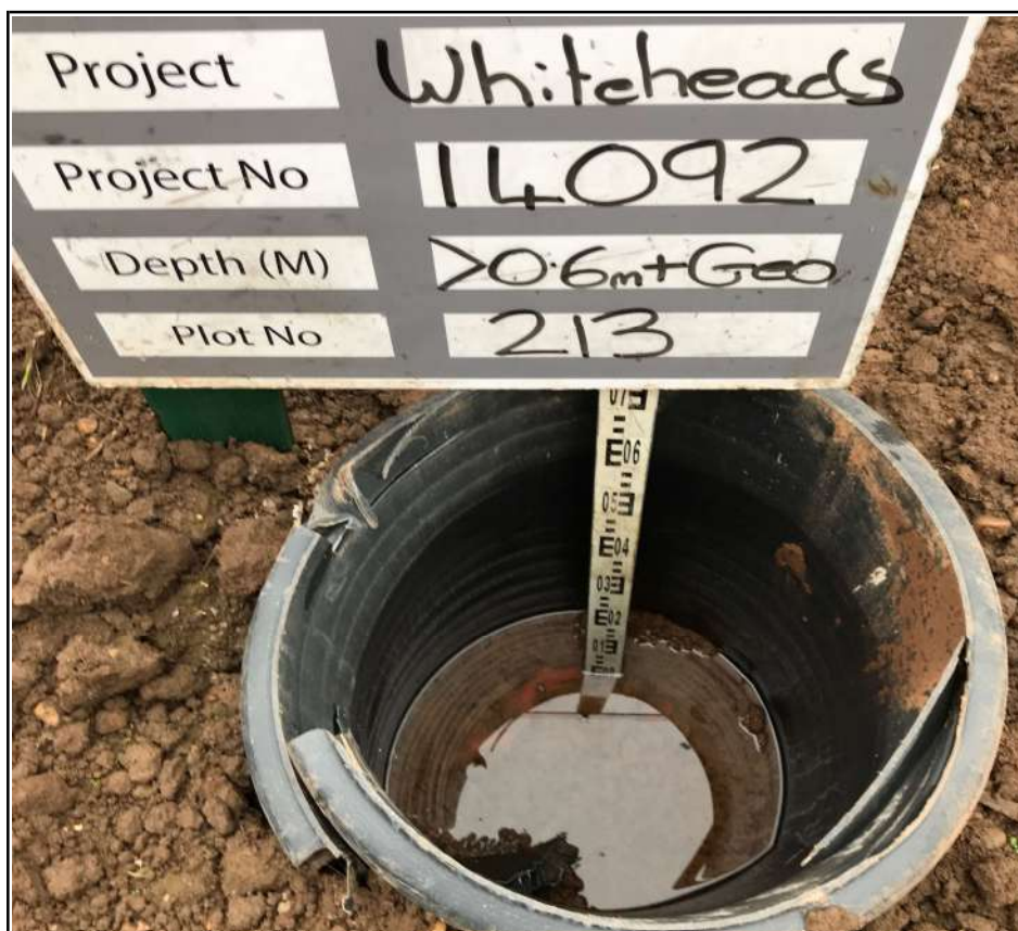
Plot 213 Membrane Placement (visable through water ingress)
