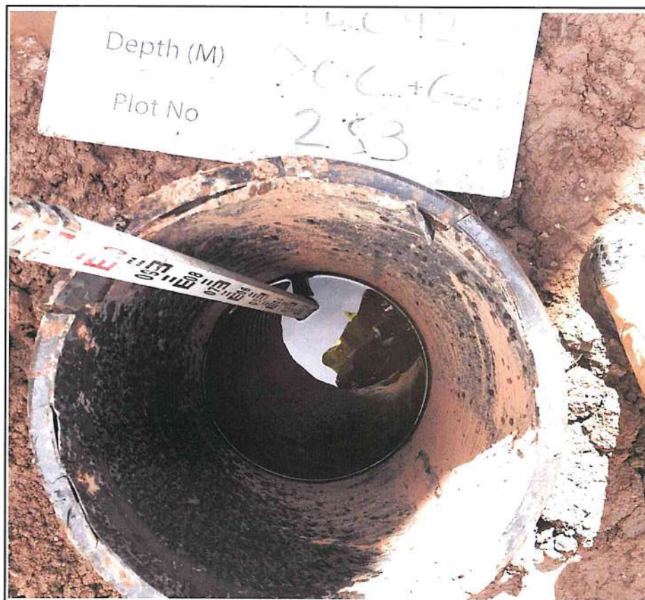
Plot 483 Membrane Placement (Membrane hand touched through Water Ingress)
