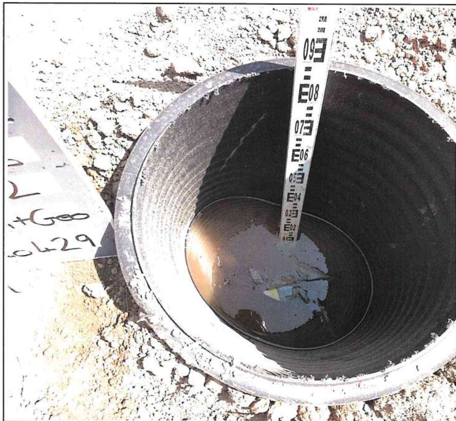
Plot 422 to 429 Membrane Placement (Visable Through Water Ingress)
