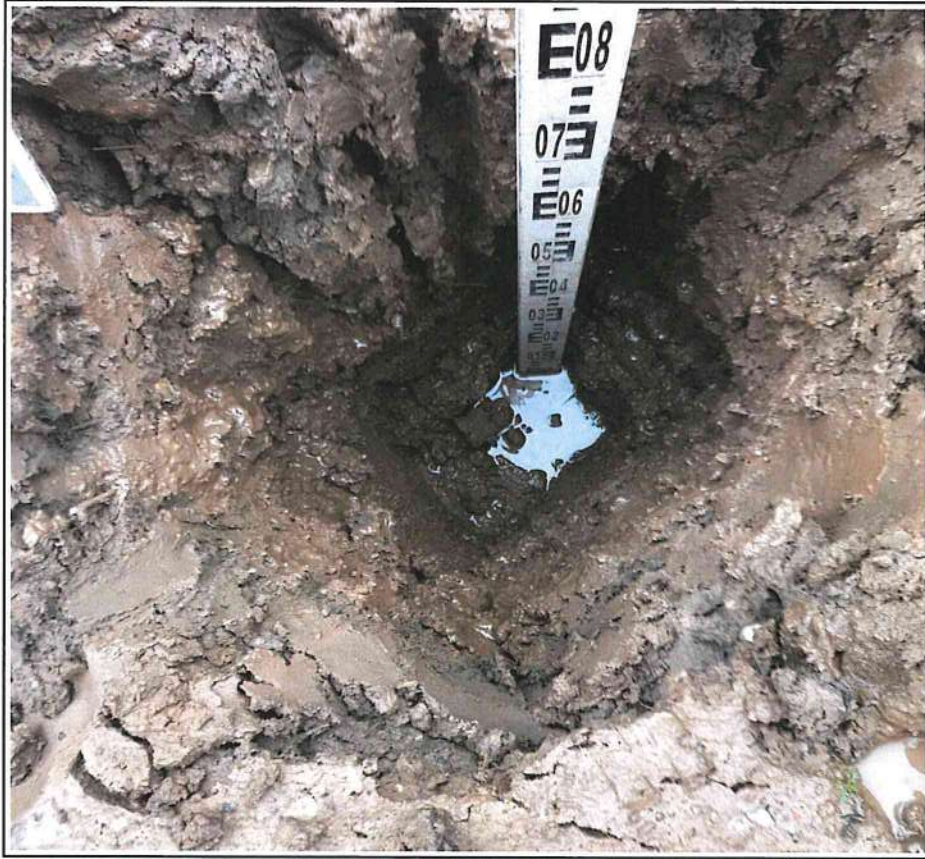
Plot 482 Membrane Placement (Membrane hand touched through Water Ingress)
