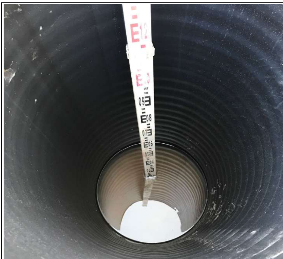
Plot 359 Membrane Placement (Hand Felt Through Water Ingress)
