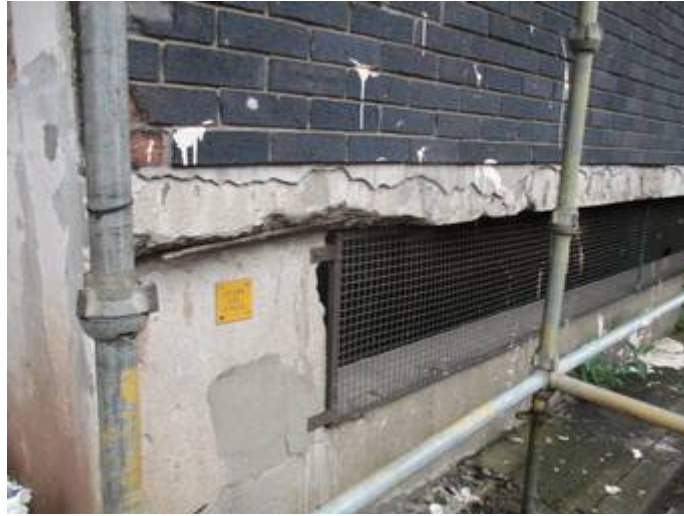
7 – A spalled edge beam/nib.
