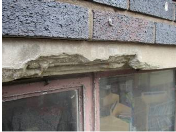
4 – View of a typical spalled edge beam/nib.
