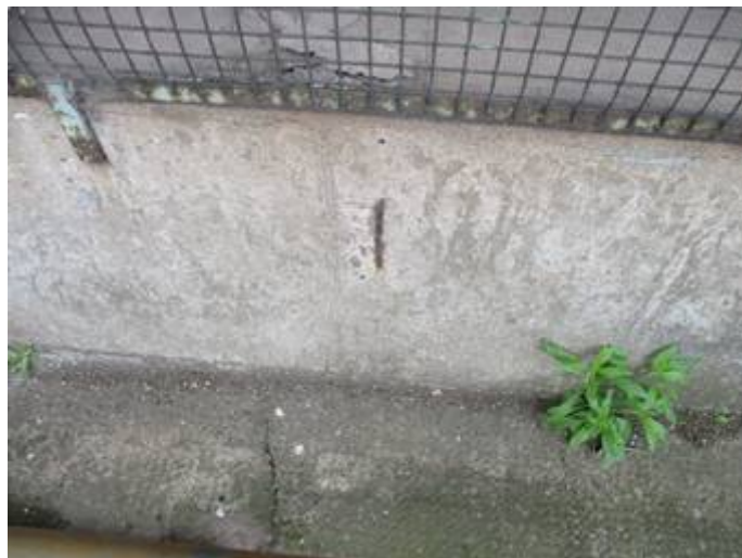
6 – A low level external spall.
