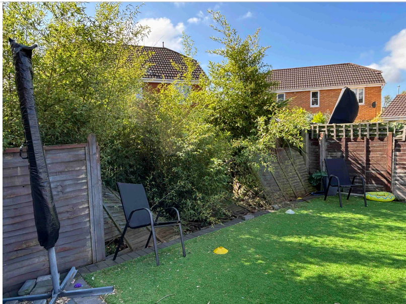
Fig. 3 Collapsed fence along boundary with number 14
