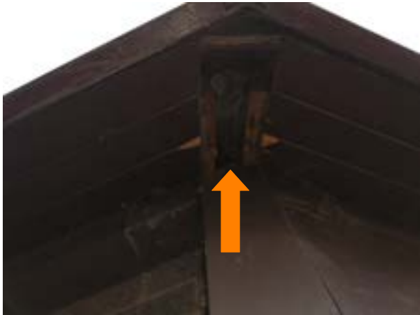
Gap in soffit
