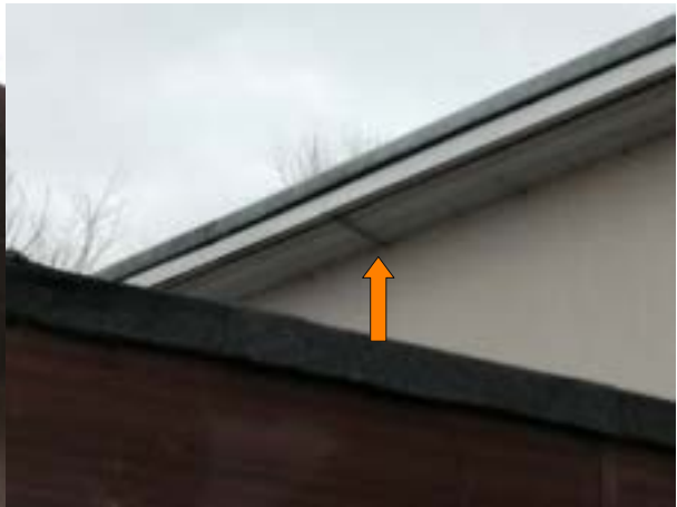
Gap in soffit
