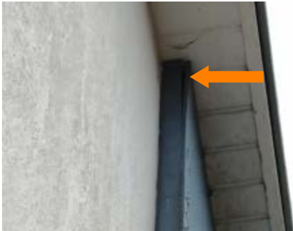
Gap in shutter casing
