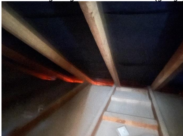
Photo 13: Light ingress within loft void 2 (garage)
