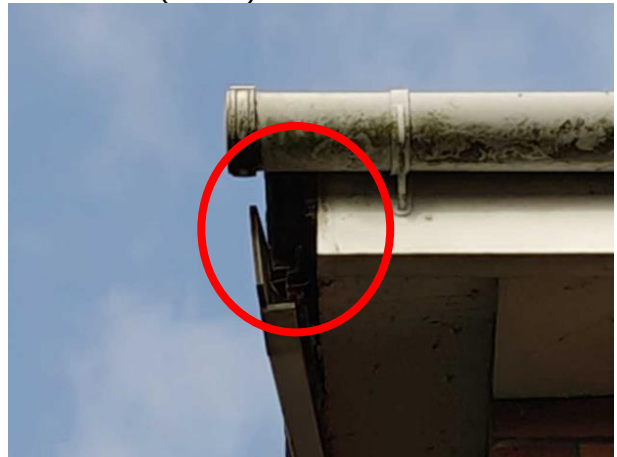
Photo 6: Gap between fascia and soffit at south-west corner (circled)
