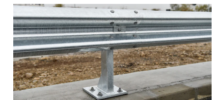
Galvanised steel Armco vehicle barrier to protect fencing adjacent to vehicle circulation routes.
