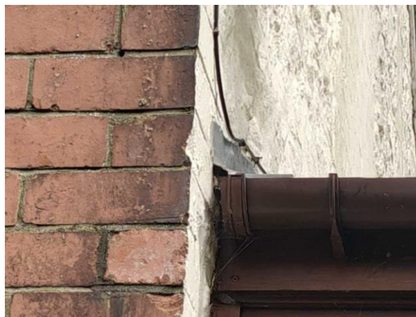
Photo 13: Gaps around the gutter.
