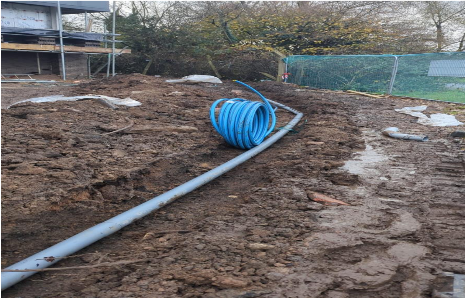
Photo 2 – The barrier pipe is the bright blue coiled pipe with typical dark blue stripe.
