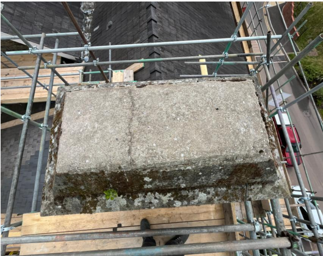
Plate 3: Top of chimney capping with crack to cementitious flaunching. Appx mortar bed depth 55mm at centre, levelling to appx 22mm at edges (finishes flush with outer edge of pylonic top stones).
